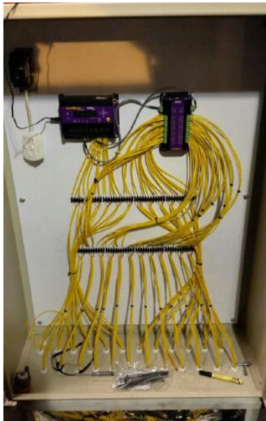
Figure 4-4: Data logger and expansion module in the protective cabinet.
