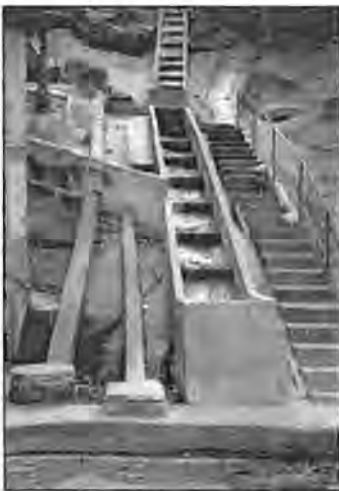
Fig. 5.7 Favela Vidigal, Rio de Janeiro: An example of services placed perpendicular to the access way in private space. Two sewers and a set of hydraulic steps for stormwater flow have been constructed alongside the pedestrian access to the dwelling on the left. The water supply pipes are just visible on the wall of the dwelling.
