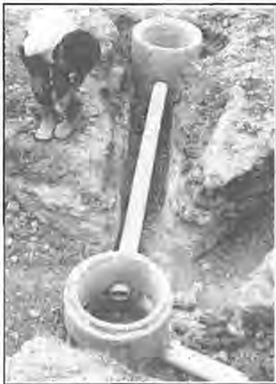
Fig. 2.20 Simple junction boxes replacing large manholes at changes in direction (Source: Mara, 1996a:132)
