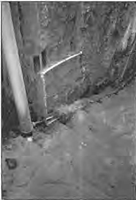
Fig. 5.8 Favela Vidigal, Rio de Janeiro: PVC water supply pipes, poorly covered with concrete, are located along the edges of this stepped pedestrian pathway. The larger pipe is a sewer that discharges into a collector sewer running down the centre of the pathway. Sewer manholes are located on the landings of the stairway at \pm 20\text{m} intervals. Stormwater flows along the surface of the steps.
