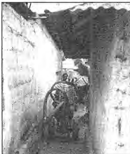
Fig. 2.13 A MAPET being used in a narrow access way in Dar es Salaam, Tanzania (Source: Mara, 1996a:90)
