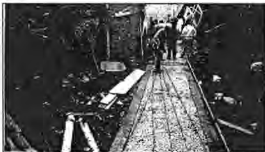
Fig. 5.17 A brick-edged, concrete pedestrian pathway being laid in a confined area (Source: M Carrilho Arquitados, 2000:134)
