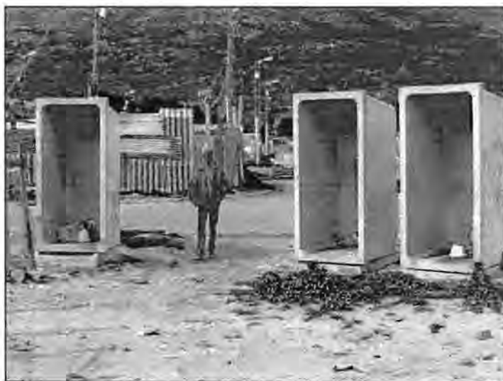
Fig. 2.1 The fate of communal toilets: A cluster of communal toilets, complete with waterborne sewers, provided in Masiphumelele settlement, Cape Town. The toilet doors and pedestals have all been removed.
