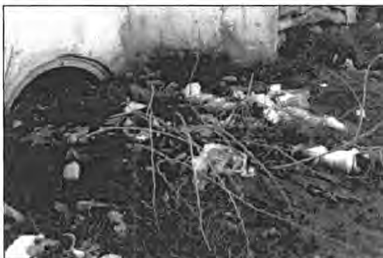
Fig. 4.3 A culvert blocked by solid waste in the Monnakato informal settlement, North West Province. (Source: DWAF, 1999)
