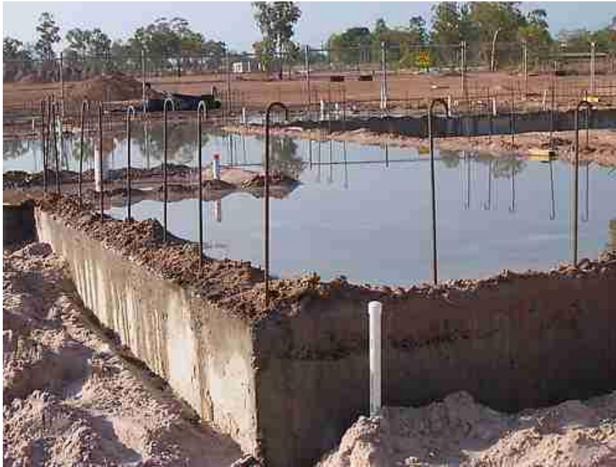
Figure 7: Ponding of water on flat concrete slab
