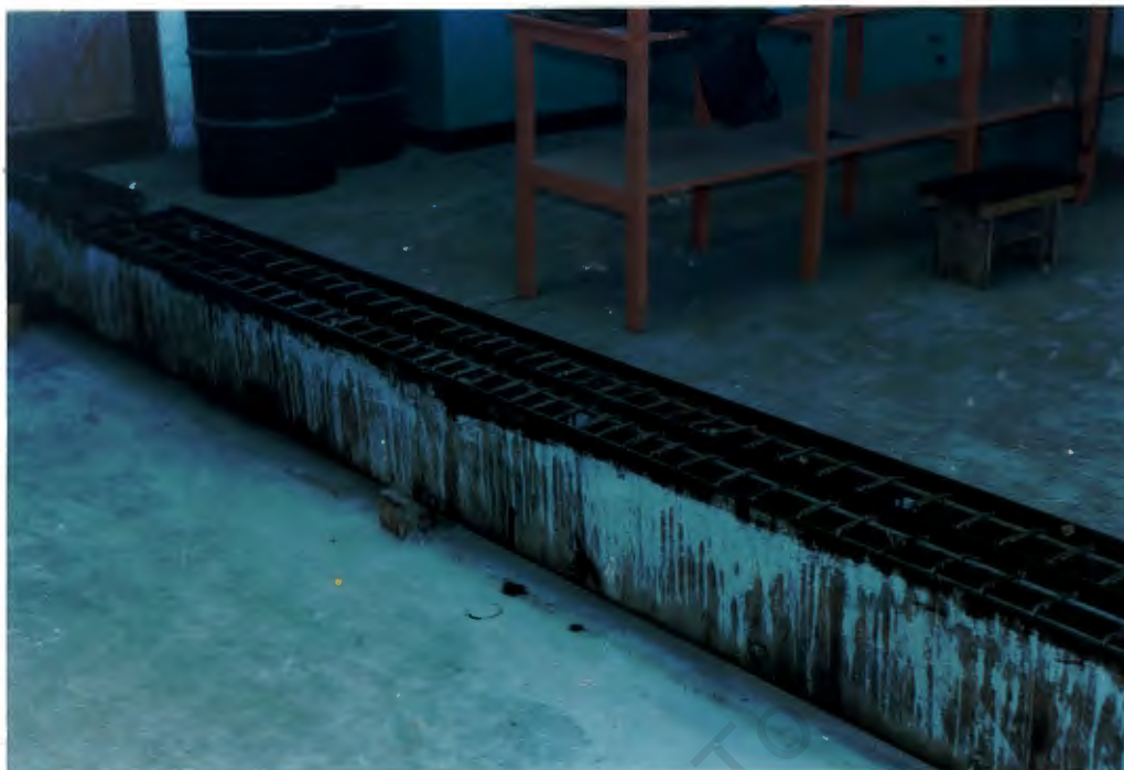
Figure 3.1: The Steel Formwork with Reinforcing Frames prior to Casting of the Concrete.
