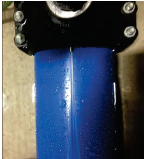
Figure 3-24: Leaking Saddle with Horizontal Circular Jet
