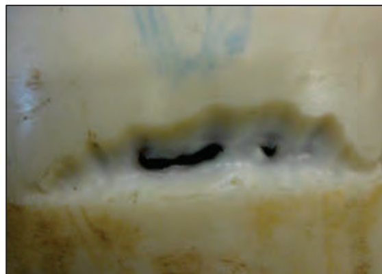
Figure 2-35: Pipe leak that has been aggravated by leakage induced erosion from the Netherlands (de Kater, 2014)
