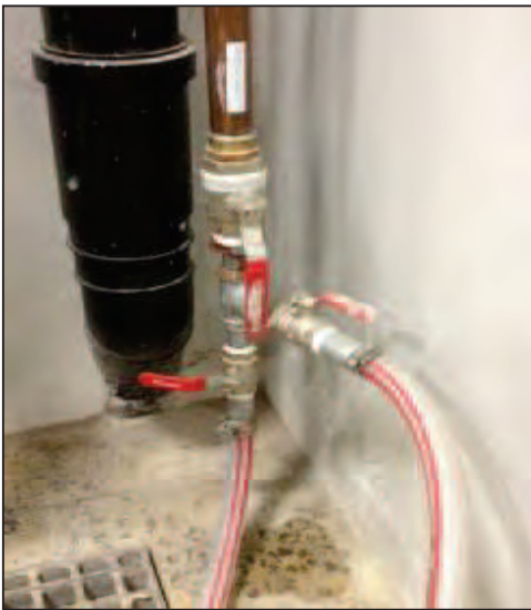
Figure 3-2: Municipal Water Supply
