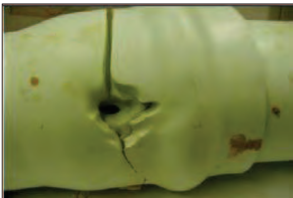
Figure 2-34: Failure in PVC-U socket due to excessive angular deflection of spigot, aggravated by erosion from pressurised leaking water (Water Services Association of Australia, 2012)
