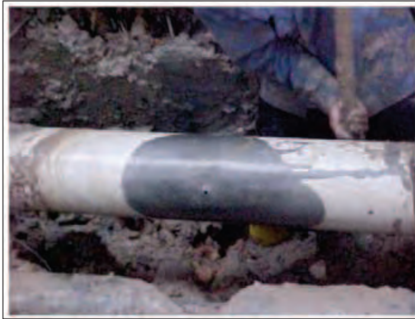
Figure 2-39: Condition of Carbon Steel Pipe Immediately after Excavation (Majid et al., 2010)
