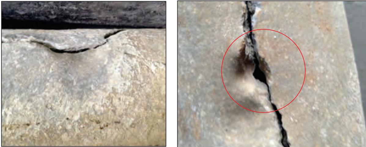
Figure 2-37: Failed Asbestos Cement Pipe Samples from The City of Cape Town (Pike, 2013)
