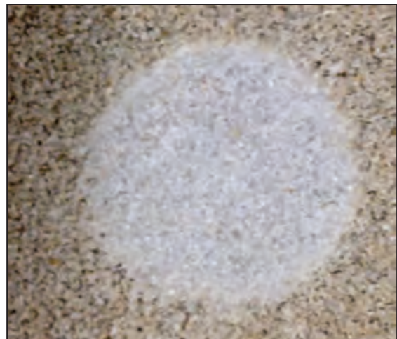
Figure 3-21: Close up view of Discoloured Region
