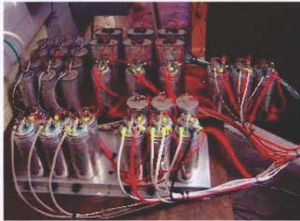
Figure 69. Photo - Additional De-rating Capacitor Banks
