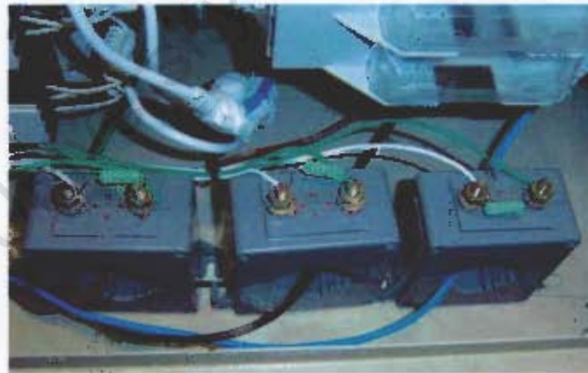
Figure 75: Photo - Unit Current Transformers
