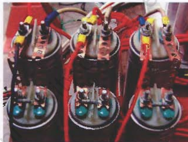
Figure 70: Photo - Connection of Additional Capacitors, Discharge Resistors
