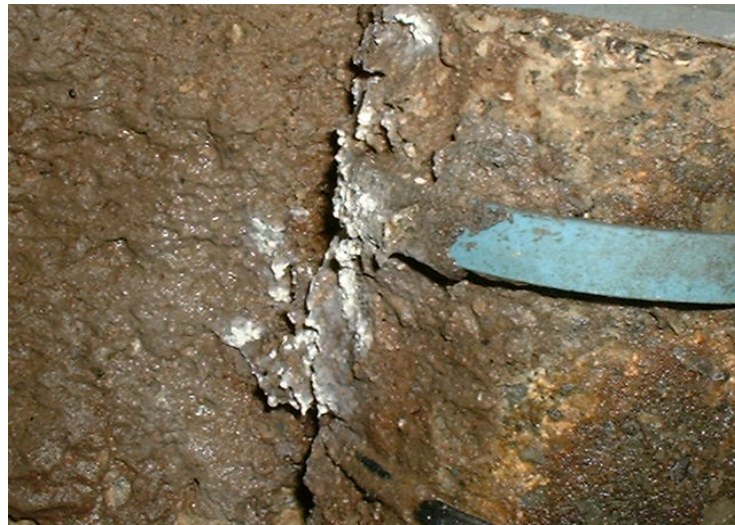
Figure 5.5 Attacked surface of concrete specimen showing release of milky white liquid on piercing of the concentrated sulphuric acid blisters
