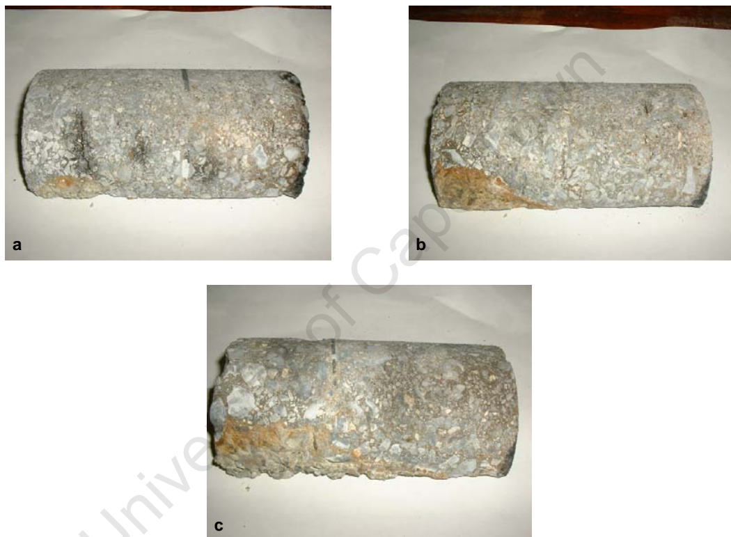
Figure 5.11 OPC/Blackheath specimens after 17 months exposure to the corrosive conditions in the manhole a) silica fume b) nickel-based biocide c) standard
