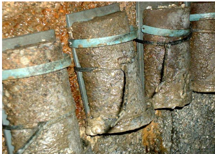
Figure 5.6 Attacked surfaces of concrete specimens 17 months after insertion
