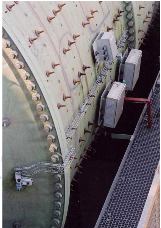
Figure 3.7 The components of the Sensomag installation on the shell of the mill
