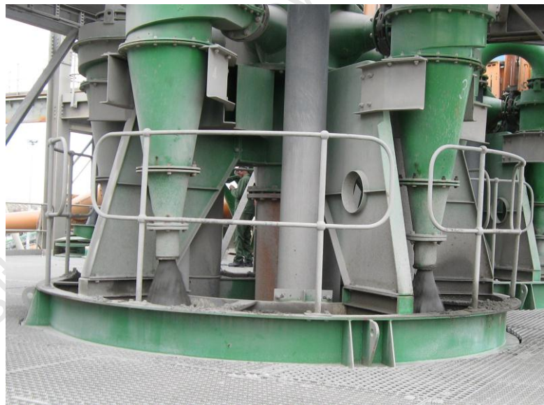
Figure 3.4 Picture of the secondary milling circuit cyclone nest at Waterval UG2 Concentrator
