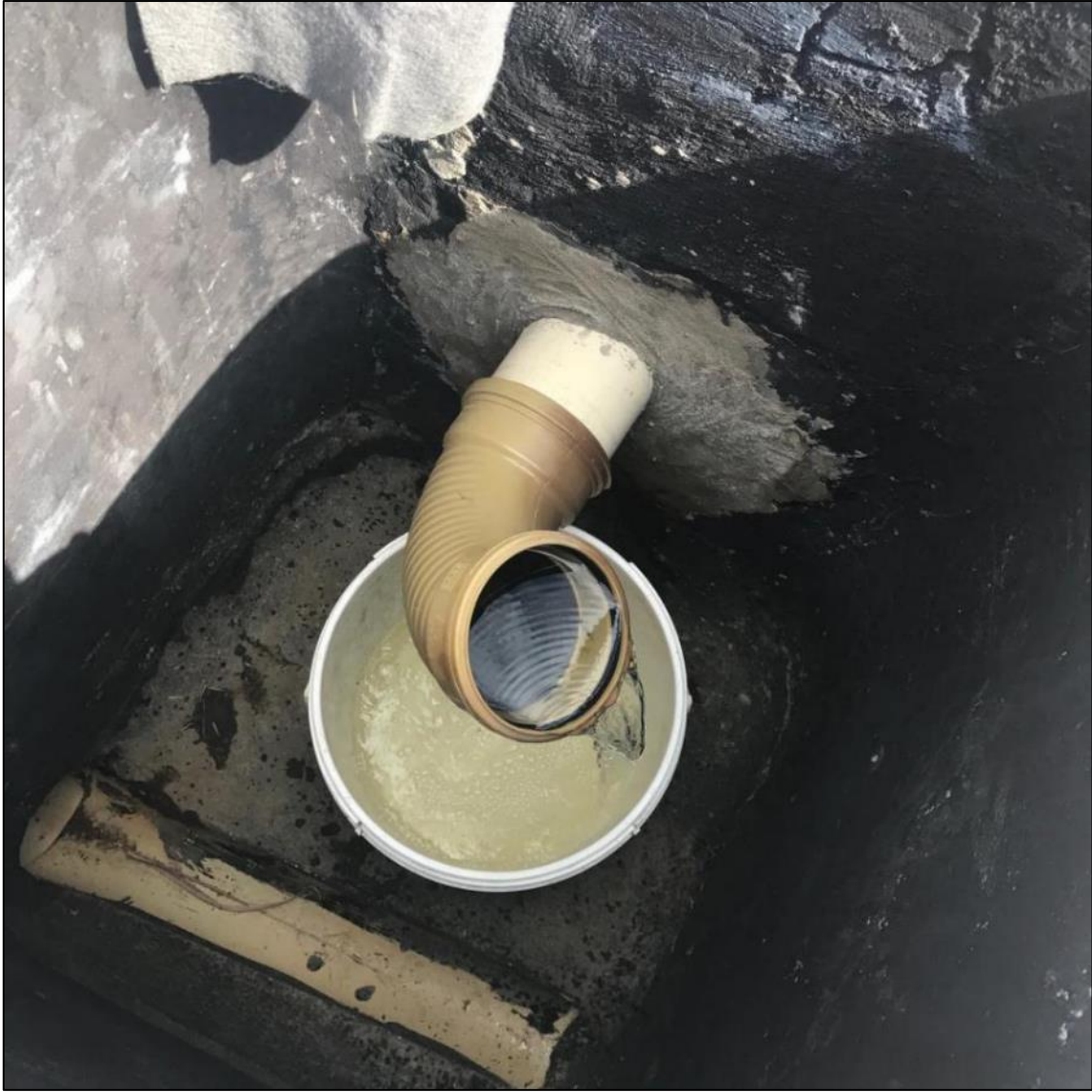
Treated water catch pit
