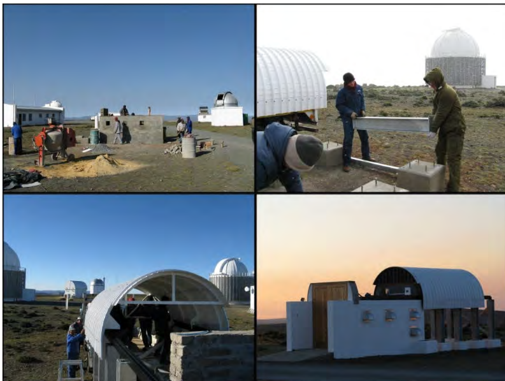
Figure 2.1: A collection of images taken during construction of the enclosure and the installation of the roof as well as the final completed building.
