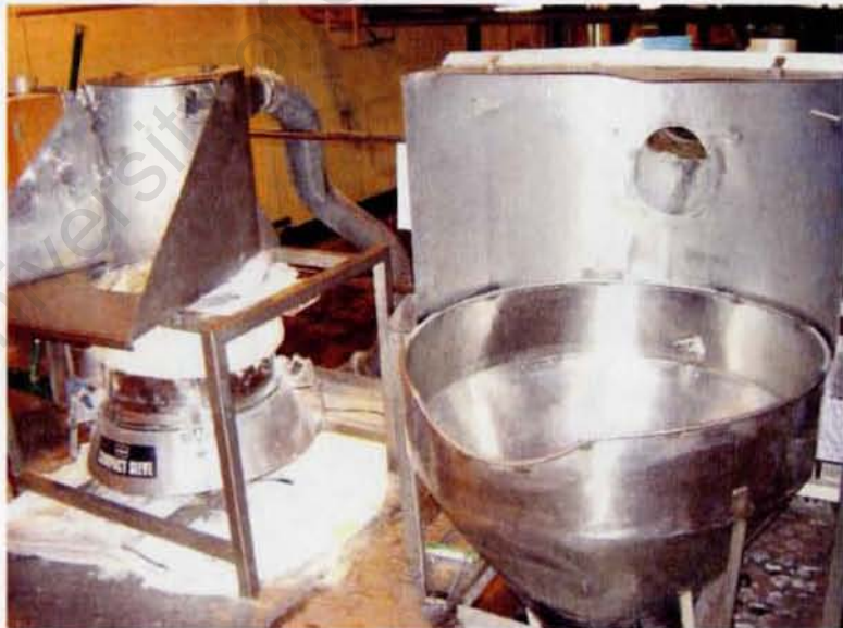
FIGURE 2: Showing typical semi-enclosed hoods provided at the charging positions of the Sifter Gantry and Blending Gantry to contain capture and remove dust before being distributed into the general working environment.
