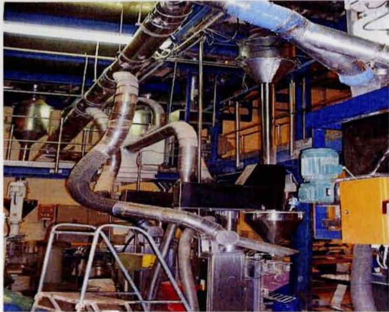
FIGURE 3: Showing the infrastructure of local exhaust ventilation (LEV) provided at packing with normal plain duct hoods at the bagging positions.
