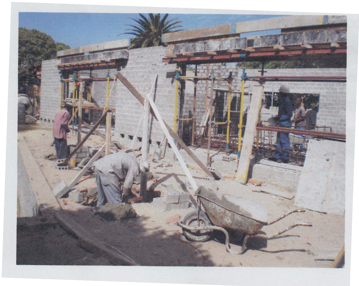
Block and Concrete Lintel under construction Source: CON 1018W 2010 Group 11 Project Report
