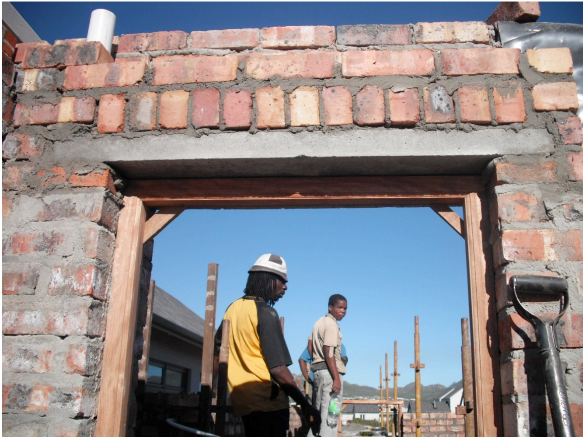
Door opening showing brick and concrete lintel Source: CON 1004W 2010 Group 8 Project Report
