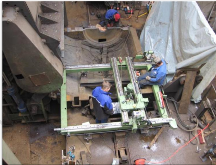
Figure 1: On-Site milling of the base of a metal shredder set in concrete foundations.
