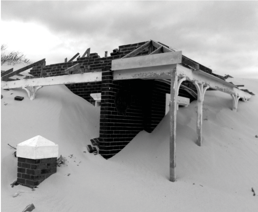
Fig 28: 2014: Buildings destroyed due to the overflow of
