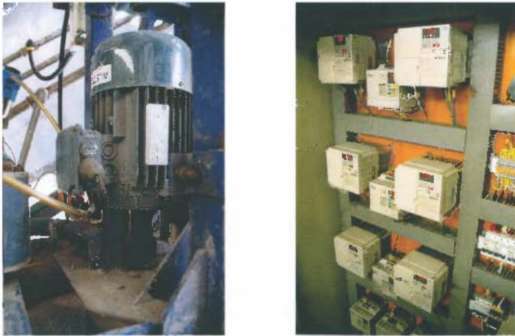
Figure 2.6 (a) Alstom 2.2kV motor, (b) Yaskawa and Omron variable speed drives.
