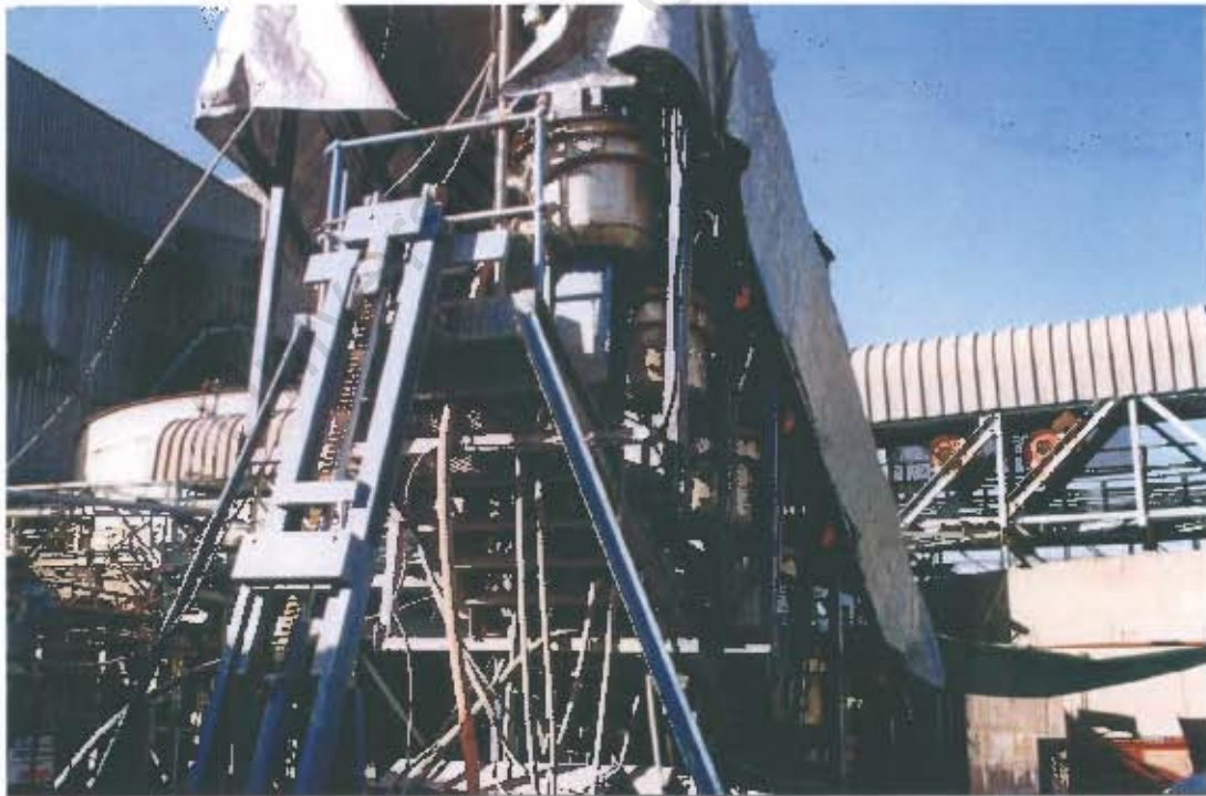
Figure 2.3 FCTR in operational position.
