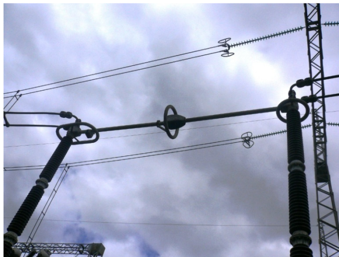
Figure 2.3 Centre side break type disconnector [Courtesy of Eskom]
