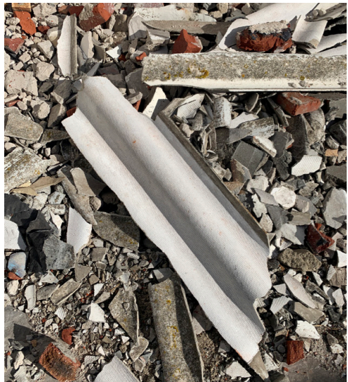
Fig. 114 - Broken asbestos sheeting lying within the rubble. (Author, 2022)
