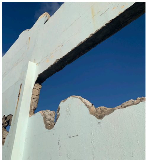
Fig. 121 - Concrete wall structure with opening (Previous window opening), framing the blue sky. (Author, 2022)
