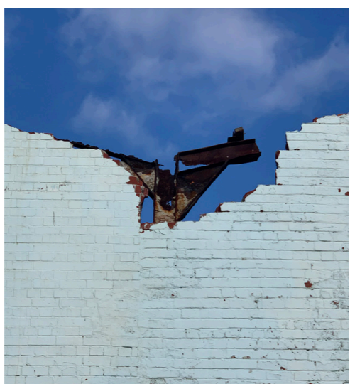
Fig. 118 - Rusted steel column and roof structure peaking out of brick wall. (Author, 2022)
