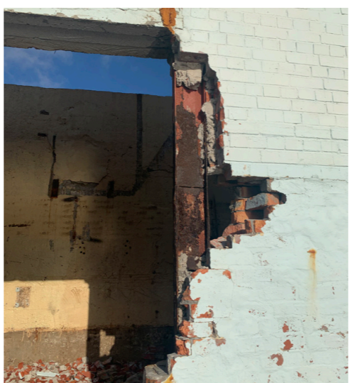
Fig. 119 - Exposed rusted steel column within brick wall. (Author, 2022)
