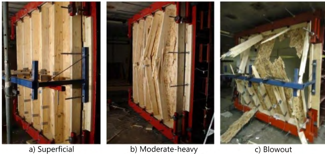
Figure 2-28: Damage observed in light-frame wood stud walls subjected to different simulated blast loads[142]
