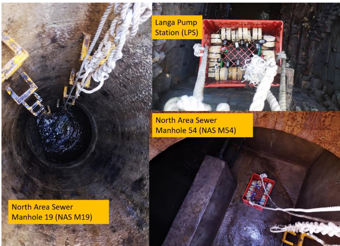
Figure 3.7: Interior appearance of the manholes involved in the study and concrete exposure
