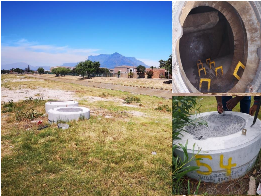
Figure 4.1: NAS M54 location in Thornton Forest drive, along the Elsiekraal River canal under the bridge. Elsie River Canal is seen in the background in the photo.
