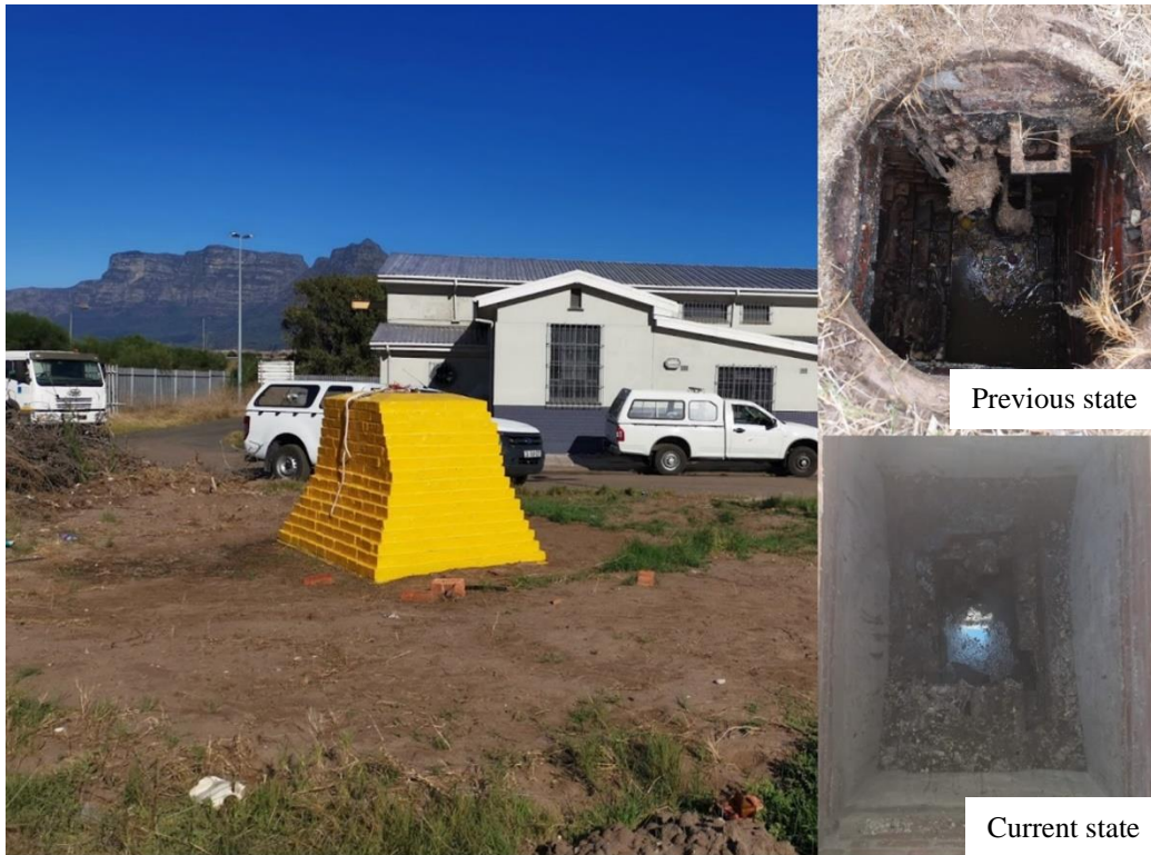
Figure 4.6: LPS manhole located between the main and minor Langa sewage pump station buildings near the Old Athlone Power Station in Cape Town. The 'Previous state' shows the sewer condition before reconstruction, and the 'Current state' shows its condition after construction. The specimens were suspended in the sewer headspace, where wastewater regularly rises and falls.
