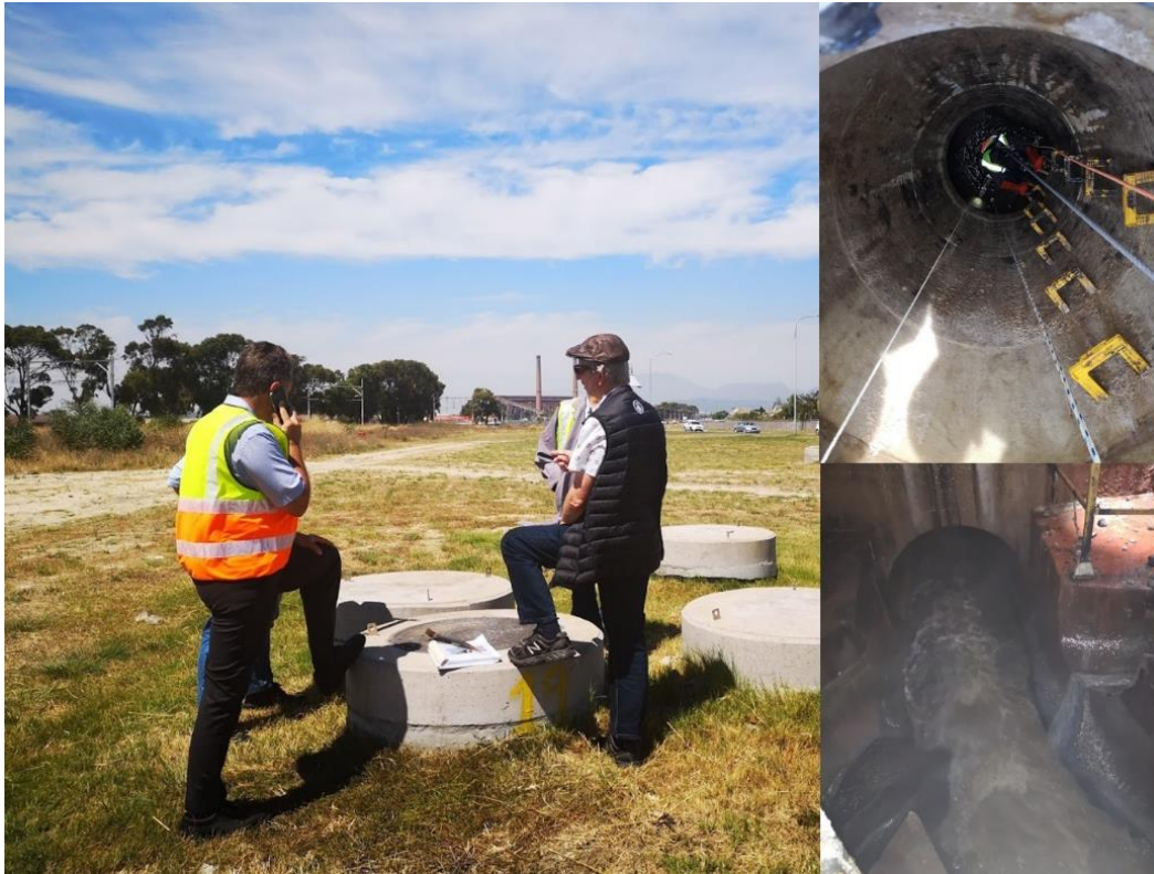
Figure 4.3: NAS M19 located along Jan Smuts Drive, near the Epping Industrial area 1 and Langa cemetery. (UCT and City of Cape Town personnel at the site).
