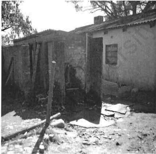
Figure 3: Dysfunctional toilets. People have to use nearby field.
