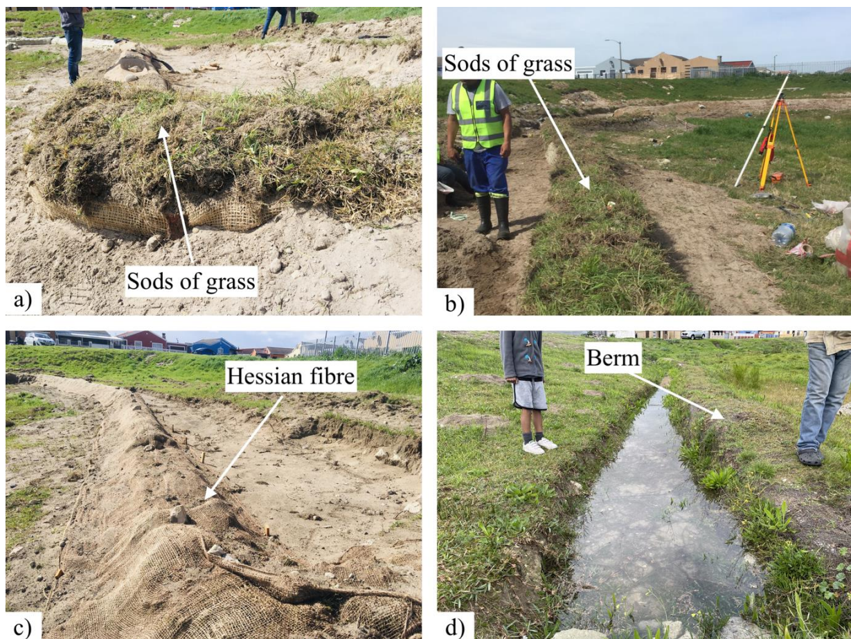
Figure 6-12: a & b) Grass placed on the berm during construction c) Hessian fibre staked to the ground d) Resident walking along the berm
