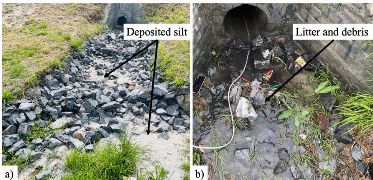
Figure 10-1: a) Deposited silt in riprap b) Riprap during after a storm
