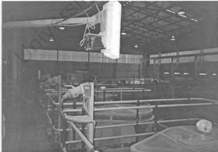
Figure 9.12: A more detailed view of the camera and floodlight assembly
