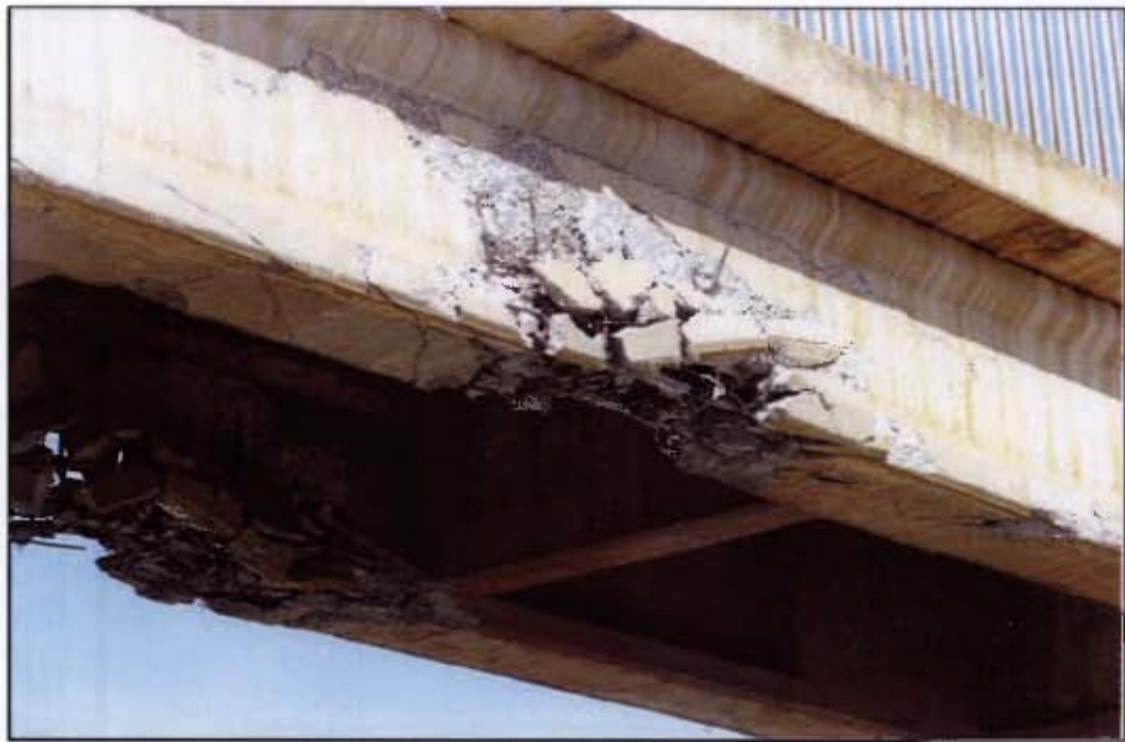
Fig 2.3: Impact damage on B267 Bridge over N1, Ackerman (2007), pp 40
