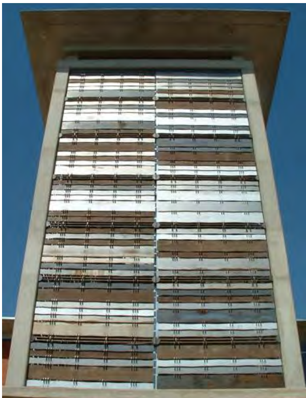
Figure 146: Metro Mall - Oxidized Steel Screens
