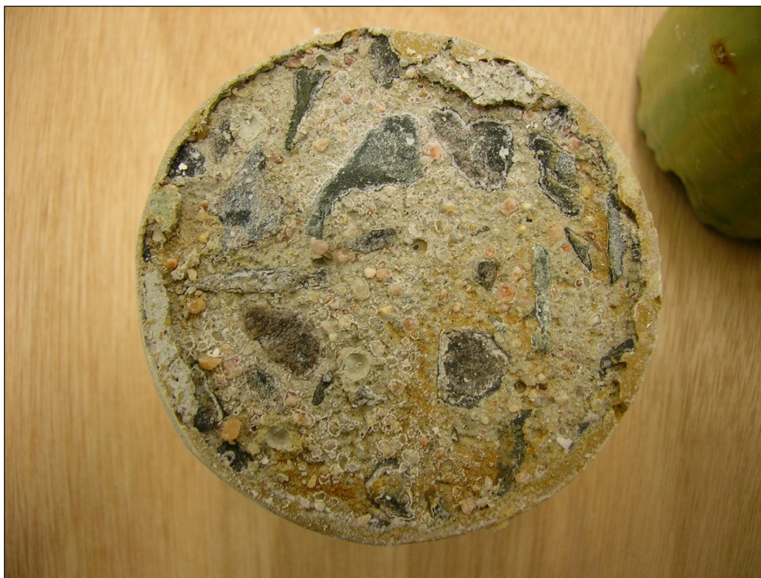
Figure 4.19: Appearance of silane/siloxane samples after the loose surface had been removed
