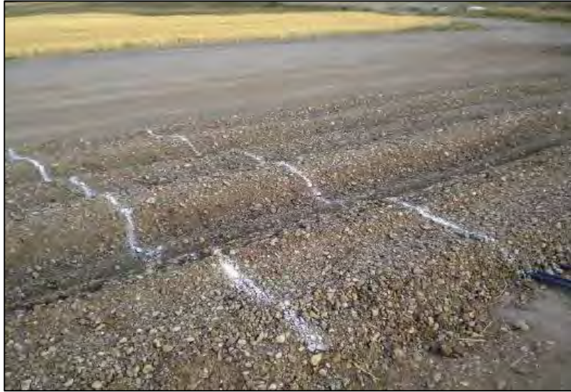
Figure 4-6: Example of the formation of rutting on a poorly designed haul road
