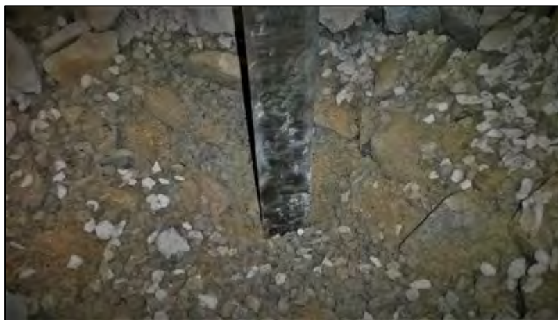
Figure 4-24: Sediment observed at different depths within Pavement C: (a) bottom of the 'lower' base 50-63mm aggregate layer
