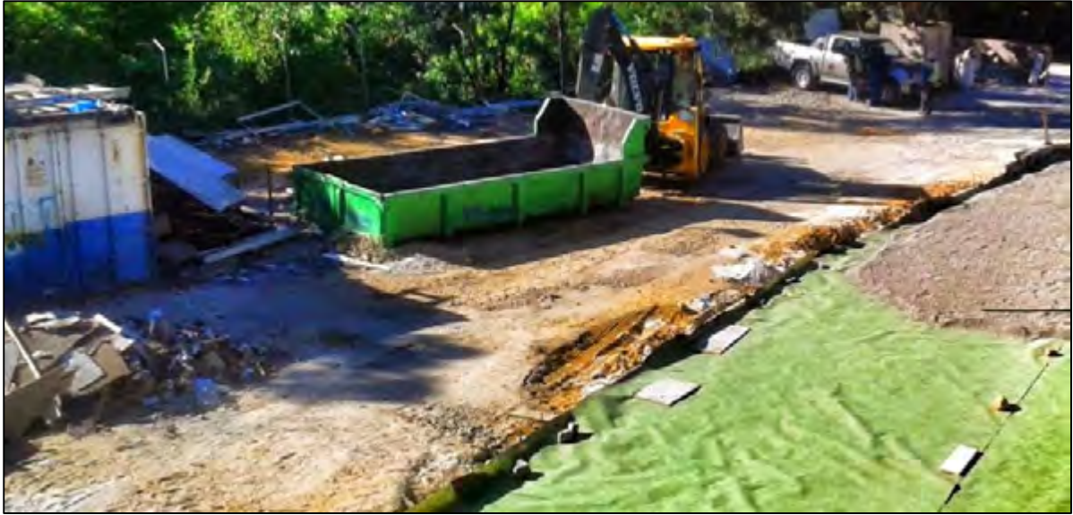
Figure D-9: Potential clogging risks are intensified by heavy machinery use
