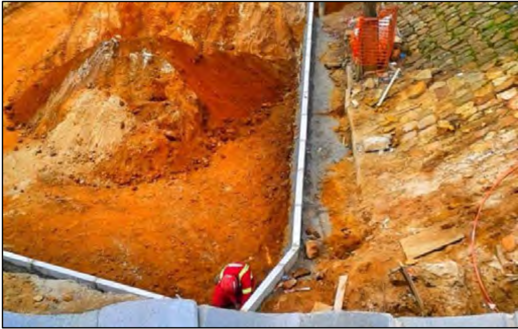
Figure D-11: Failed embankment on the site causing pollution of the pavement
