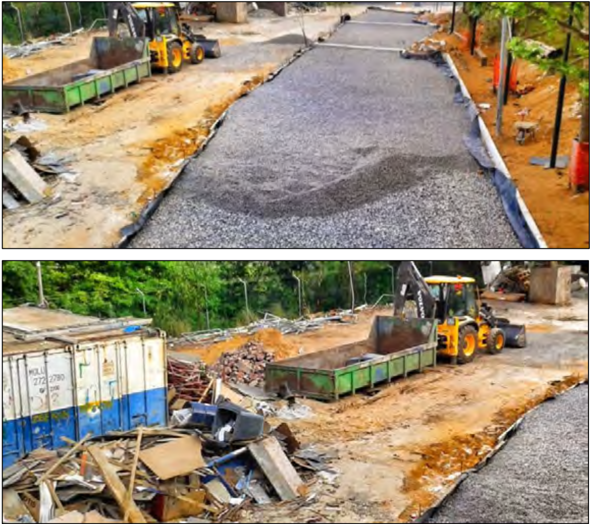
Figure D-8: Clearing of rubble with heavy machinery adjacent to sub-base stone layer
