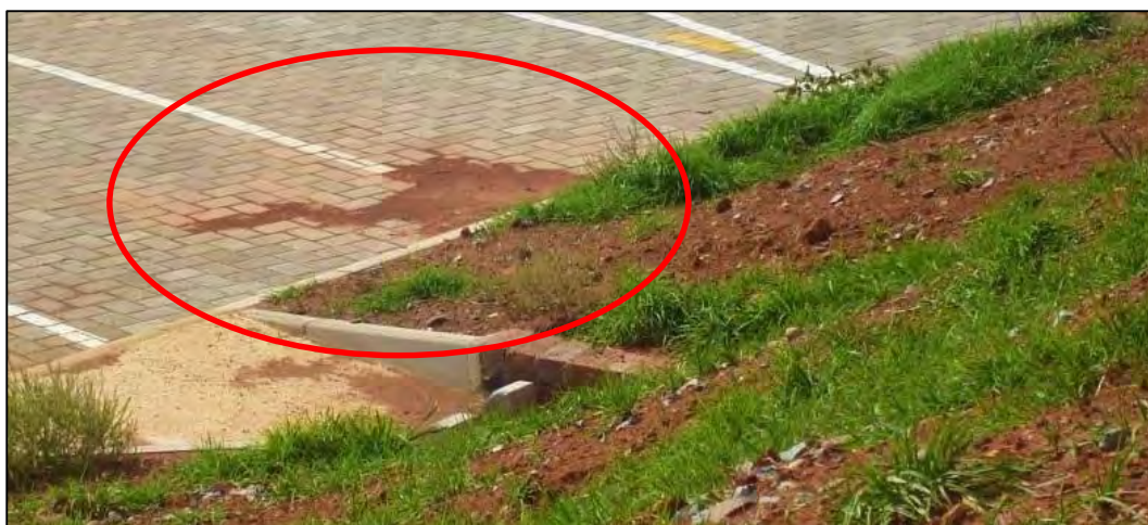
Figure 2-18: Soil embankment located adjacent a PPS causing surface clogging (Voogt, 2011)
