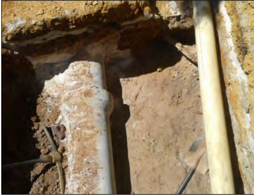
Figure D-4: Excavation of monitoring chamber B down to the existing stormwater pipe
