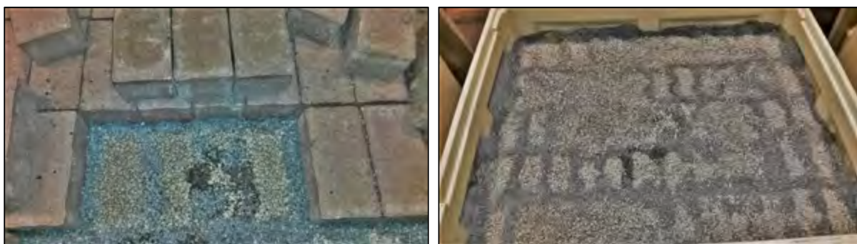
Figure 4-19: Oil stain on the bedding layer directly below the pavers
