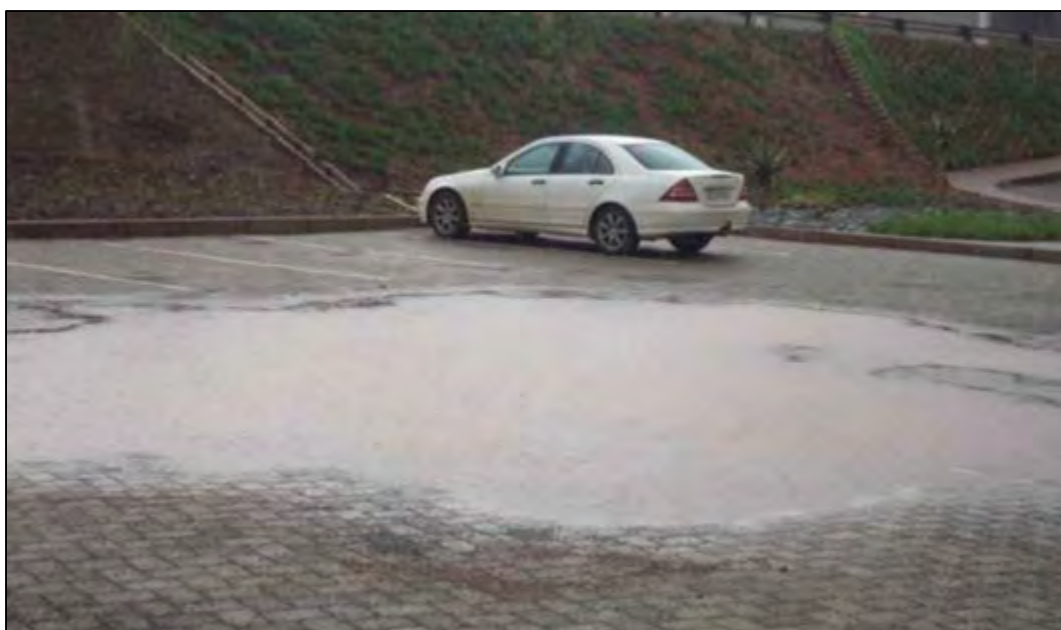
Figure 2-16: Surface ponding on a section PPS indicating pavement failure (Voogt, 2011)
