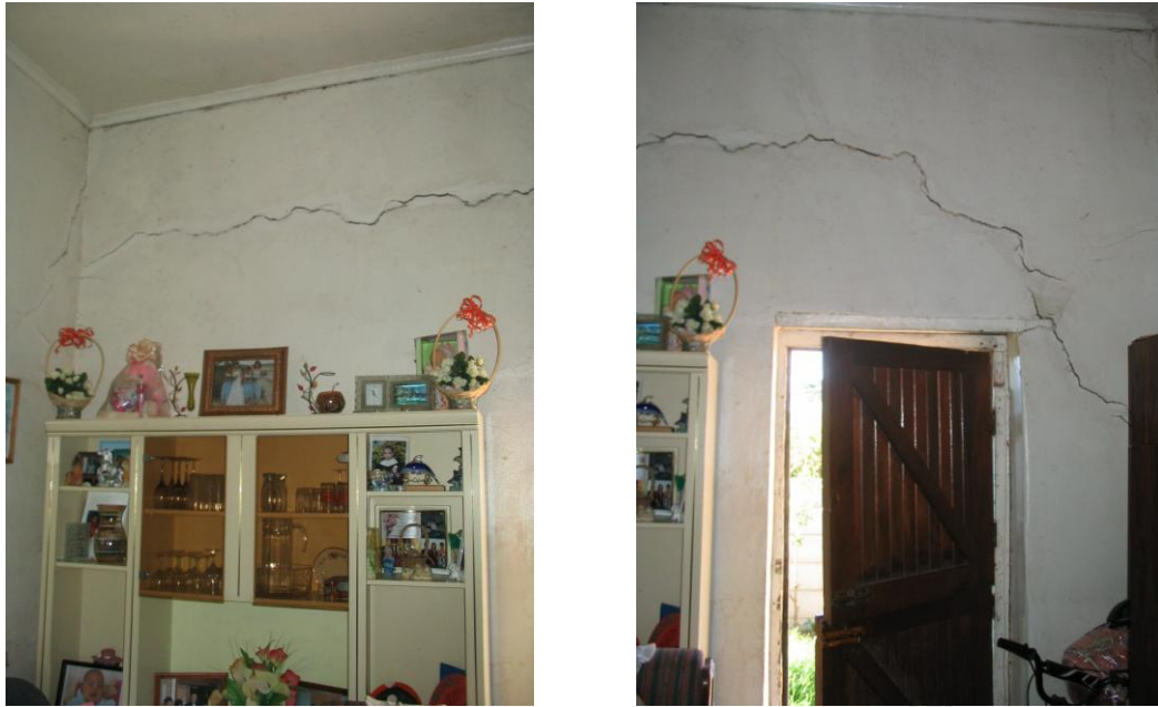
Fig 24: Internal view of crack running through the northern wall of the dwelling on Erf 285.
