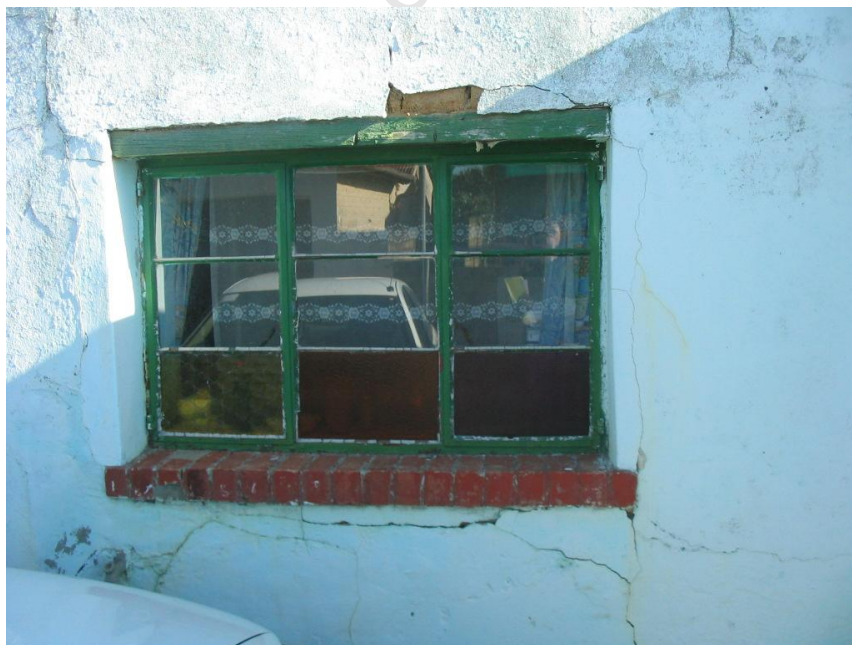
Fig 17: Modern steel window frames, brick window cill and old timber lintel above
