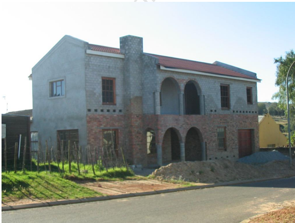
Fig 27: Double storey building under construction around the corner from both Incidents. Is this what is desired? What does it say about perceptions of significance? (Own photograph, 2010)
