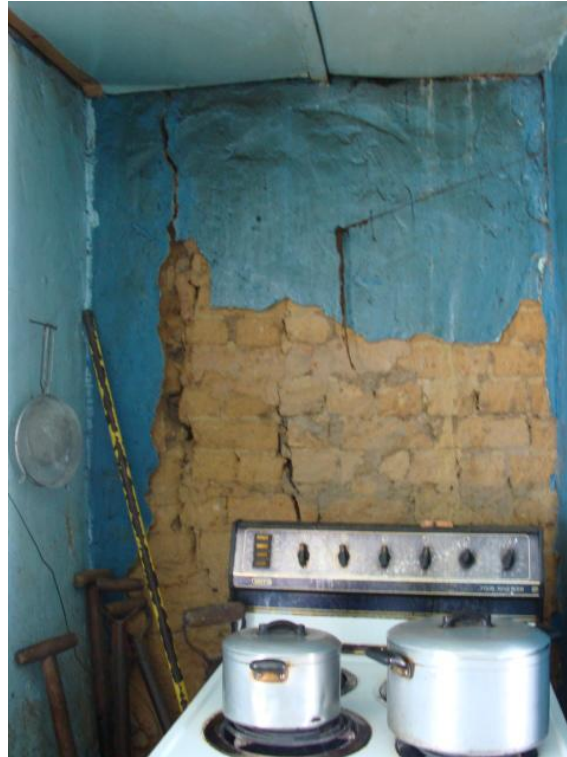
Fig 28: Internal fabric plastered over and painted. A board ceiling has also been installed below the original reed ceiling.
