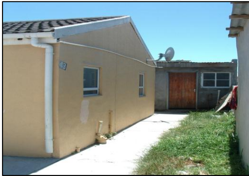
Figure 39a: Guttering without drains
