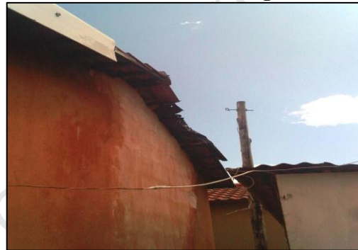
Figure 14b: Incomplete roof (Better Life, October, 2010)
