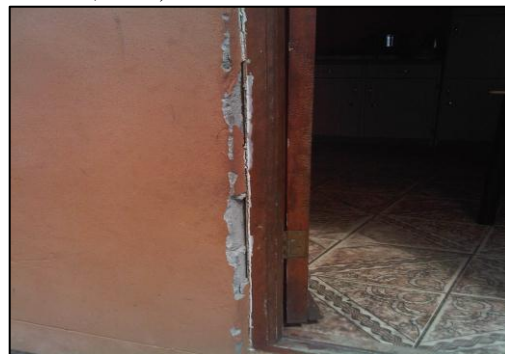
Figure 14d: Cracking around a door frame (Better Life, October, 2010)
