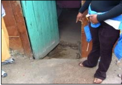
Figure 4e) An illustration of seepage or upwelling due to a high water table ('rising flooding') (Khayelitsha, June, 2006)
