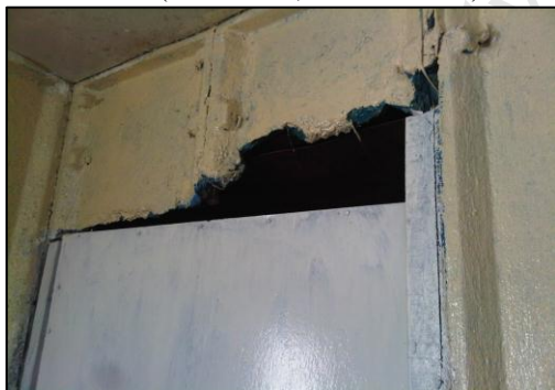
Figure 14c) Hole in a concrete wall panel (Samora Machel, November, 2010)
