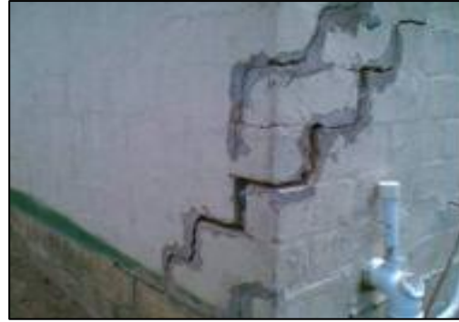
Figure 4f) An illustration of leaking walls (Thembaletu, August 2006)
