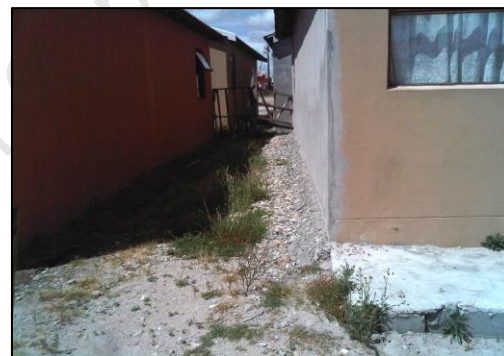
Figure 30b: Dwelling with a re-plastered wall (Better Life, October, 2010)
