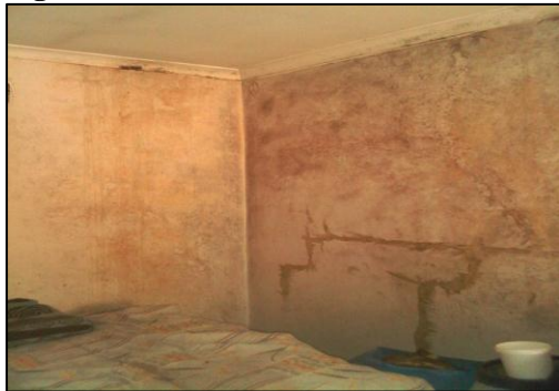
Figure 14a: Structural cracks and damp in an internal wall (Better Life, October 2010)
