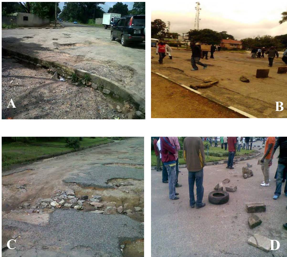
A and C show the poor state of roads in Chingola. B and D show residents blocking roads during a protest in Chingola. Source: Mubanga Chileshe and social media
