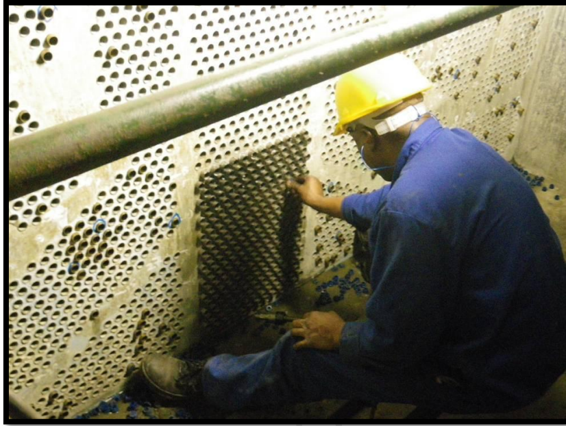
Figure 2.2: The inside of a water box at a power station. The condenser was in the process of being re-tubed.
