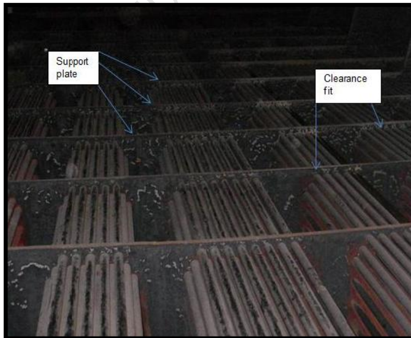
Figure 2.3: Condenser steam space showing the tube bundles and tube support plates.
