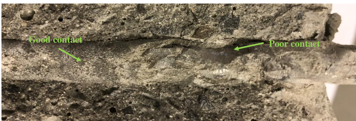
Figure 45: 20% corroded coated steel after failure
