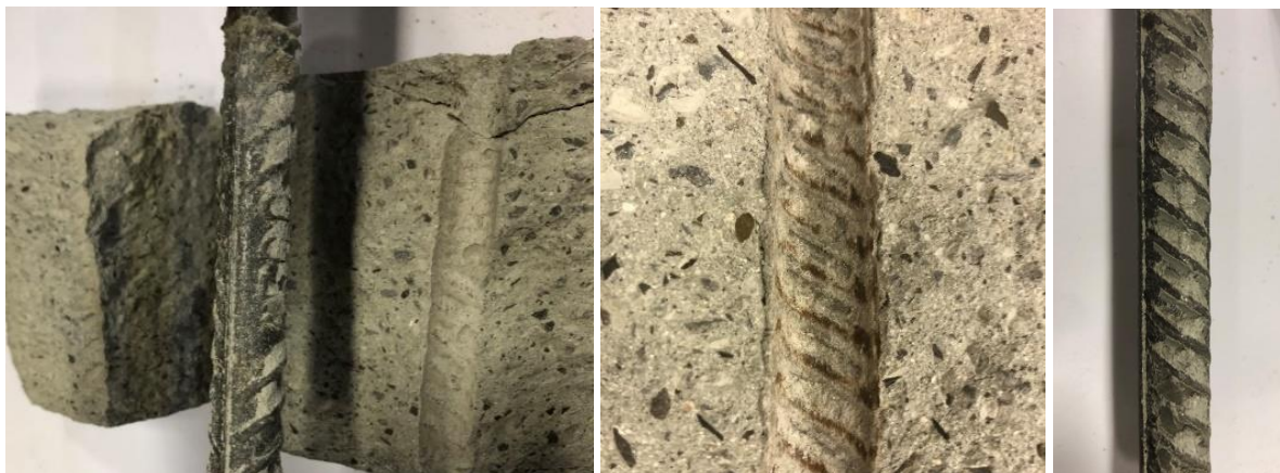
Figure 35: Coating failure with 10% corroded steel
