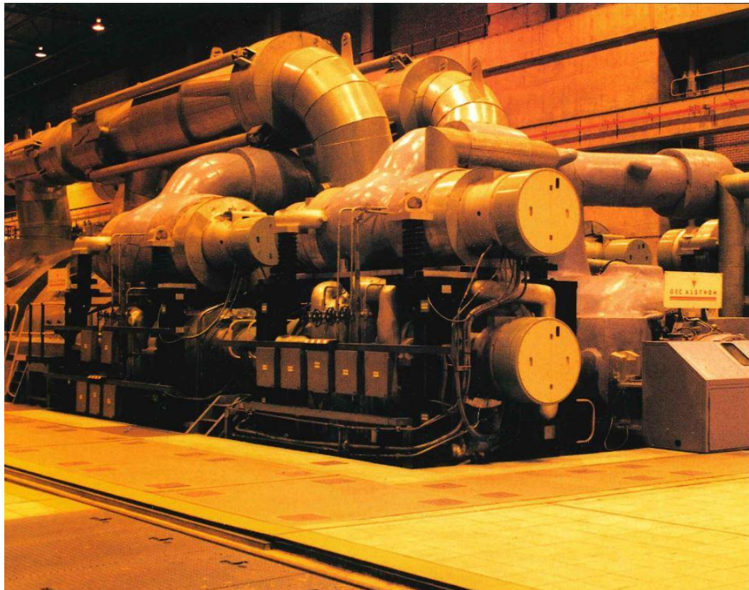
Figure 3: HP turbine at Majuba Power Station [16]
