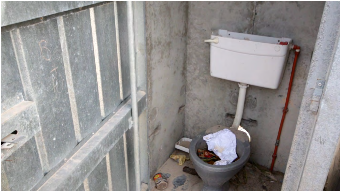
Figure 2: A blocked full flush toilet in Enkanini, Khayelitsha. Photo: Shaun Swingler
