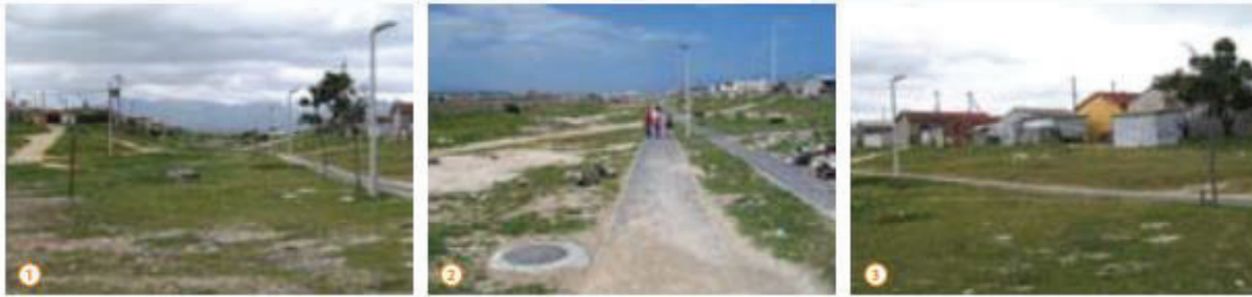
Figure 92 Some parts of the cycle path are situated in a depression, thus further compromising the safety of cyclists and pedestrians
