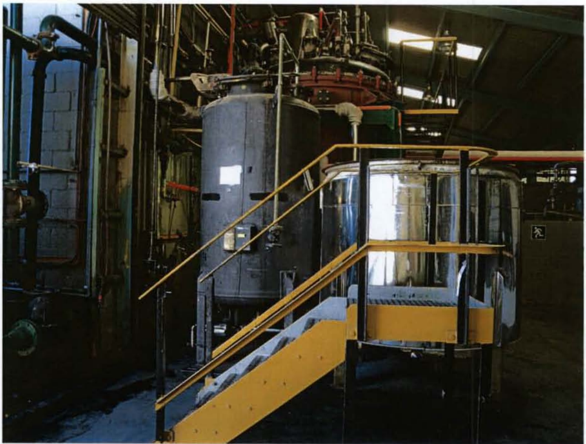
Figure 3.8 Phenol resin tanks
