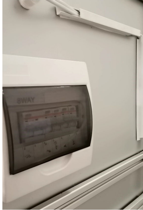
Figure A15 - Distribution Board
