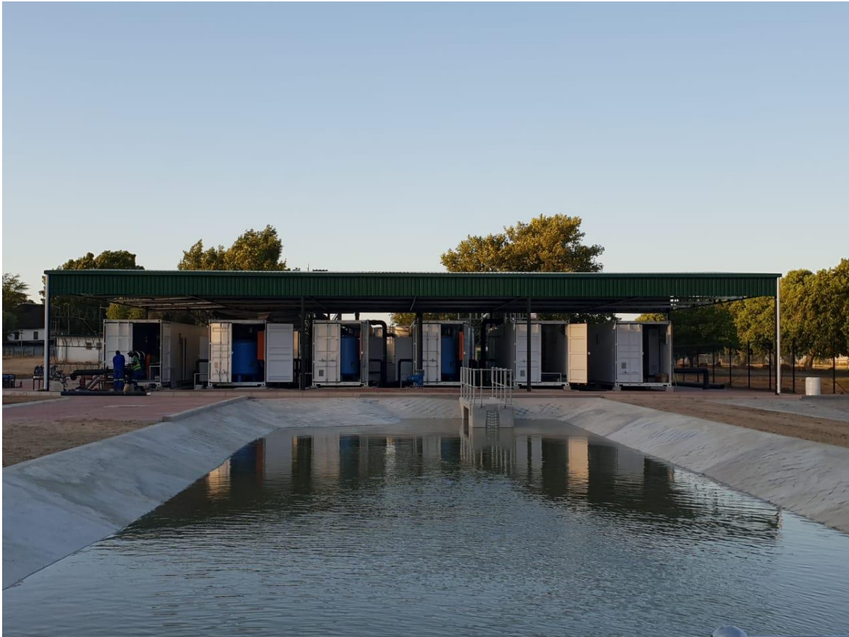
Figure 4-2: Final groundwater abstraction water treatment plant at Boy Louw Sportsgrounds
