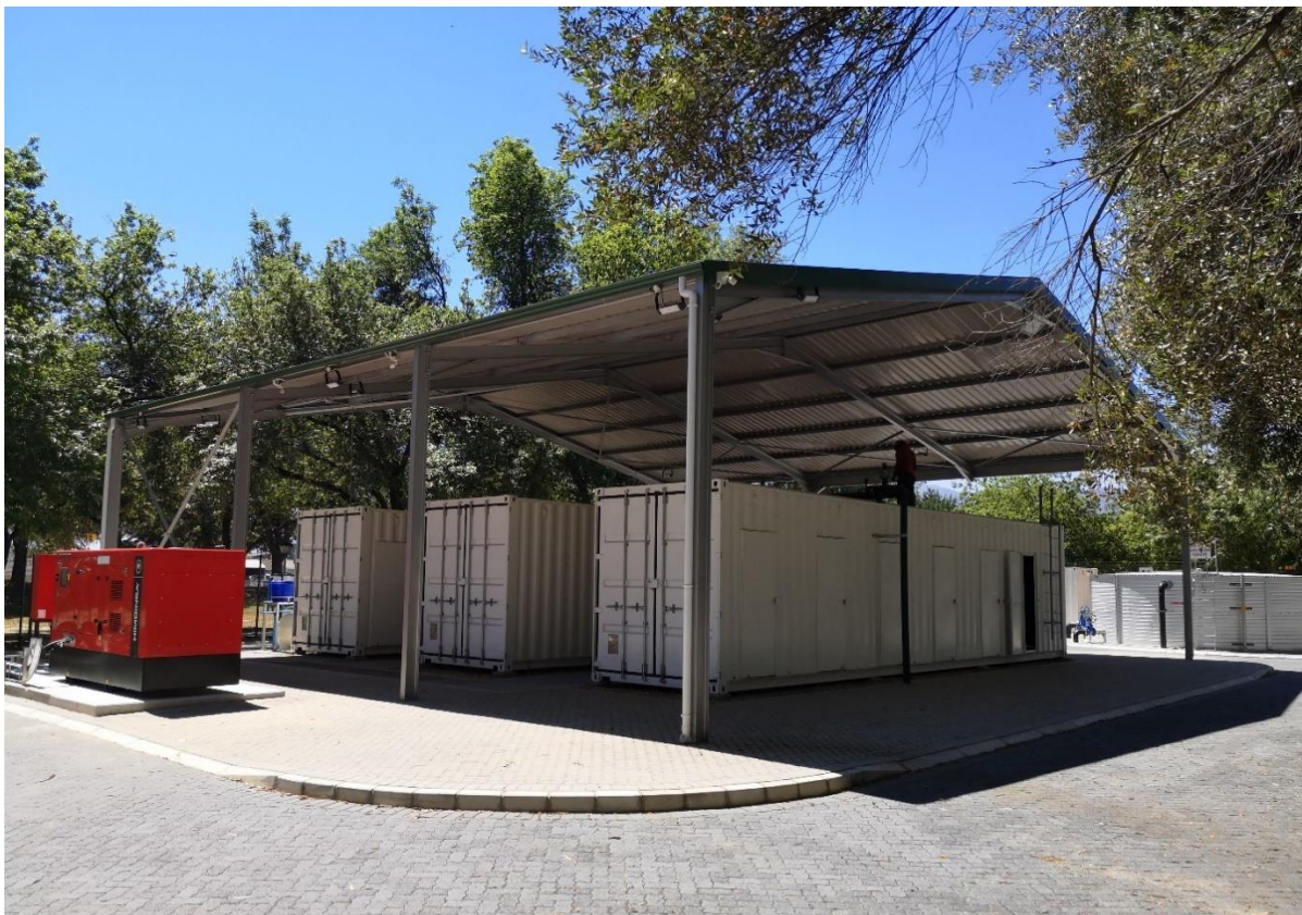
Figure 4-4: Final groundwater abstraction water treatment plant at Parys Sportsgrounds
