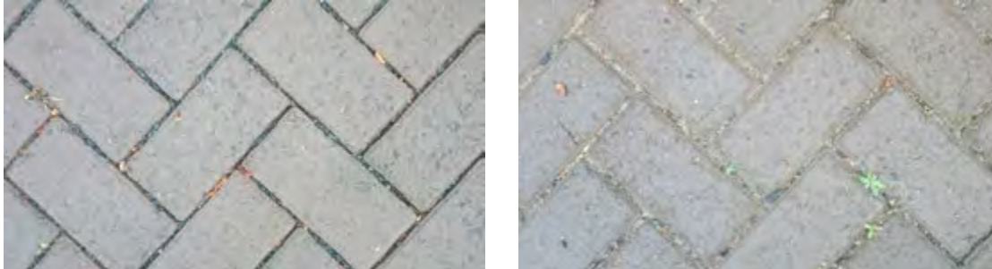
Figure 6-2: NEB Pavers nearer the centre remain clear after one rainfall season (left). However, pavers near the rain garden are filled with sediment (right)
