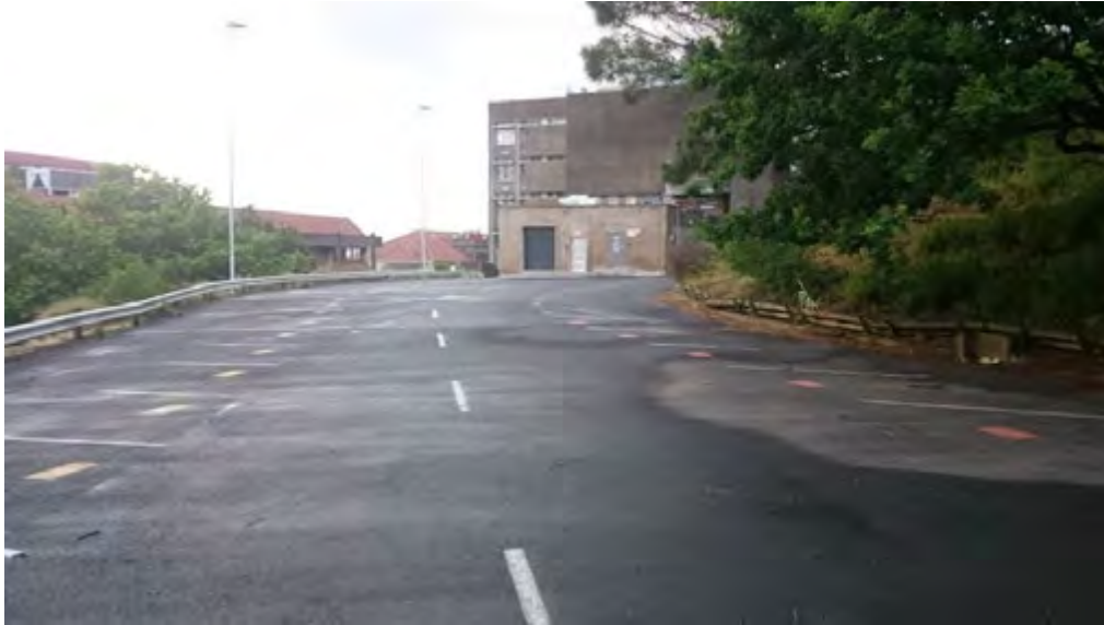
Figure 3-10: Picture of P8 shortly after rainfall. Runoff discharges into an open culvert on the left of this picture
