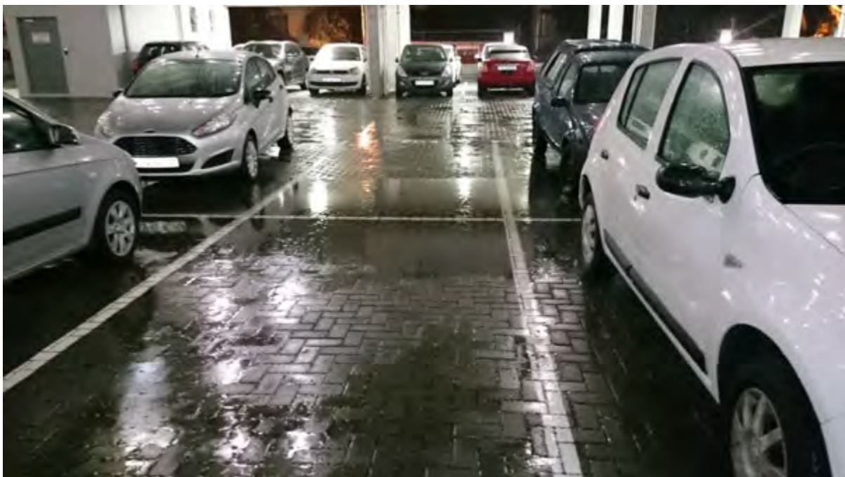
Figure 6-1: RPPS during rainfall. Note the ponding in the centre of the pavement
