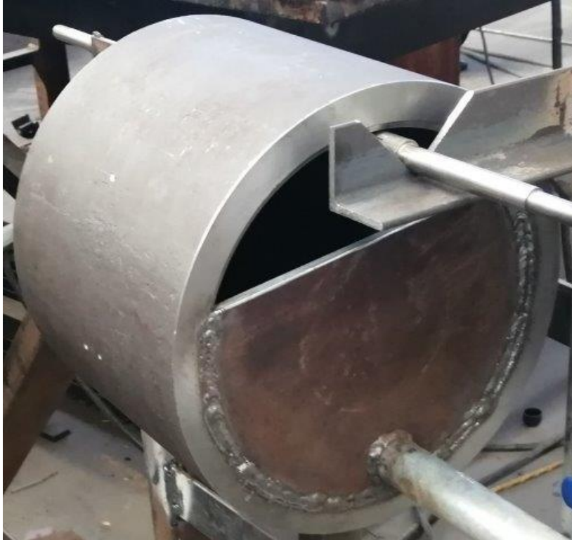
Figure 96. Steam pipe section during fabrication showing endplate, support and water admission pipe
