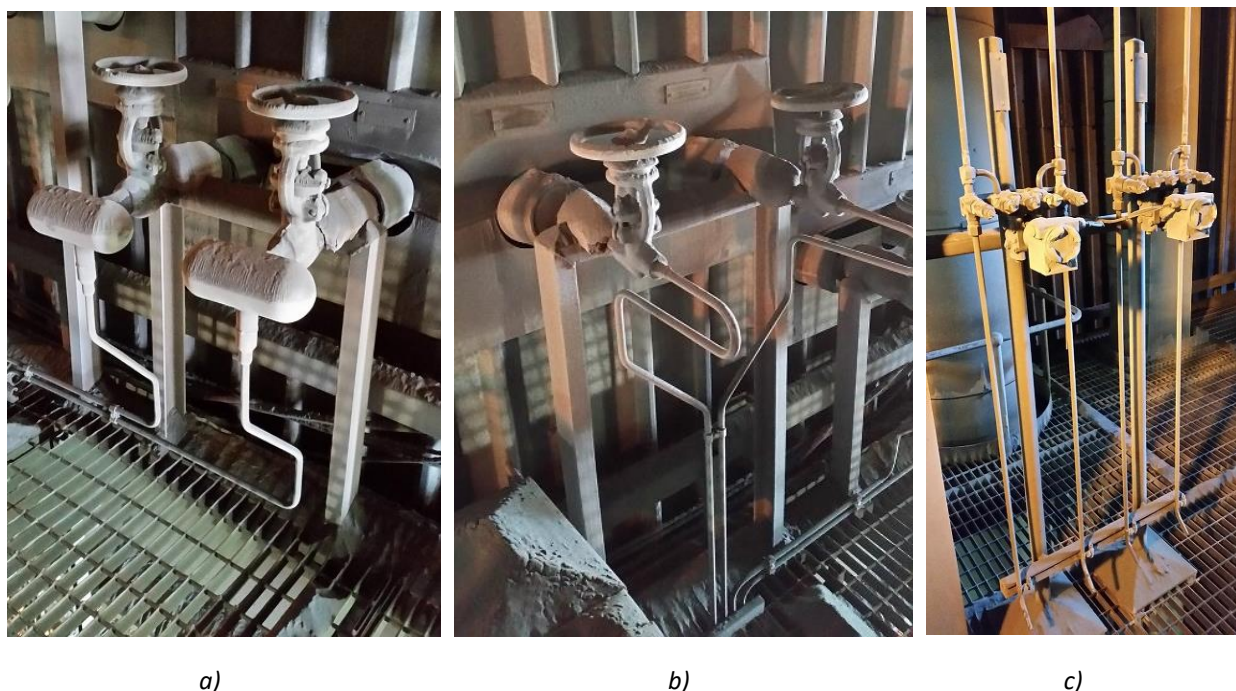
Figure 132. Collecting vessel level measurement a) Upper tapping points b) Lower tapping points c) Pressure transmitters
