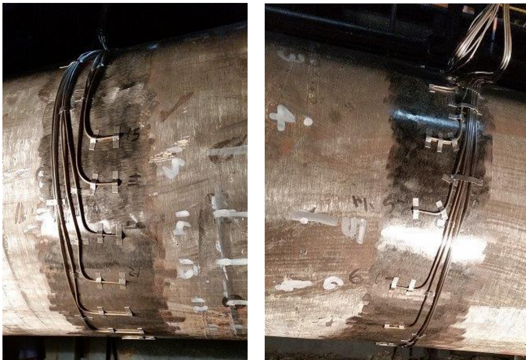
Figure 118. Thermocouples installed around the circumference of the pipe
