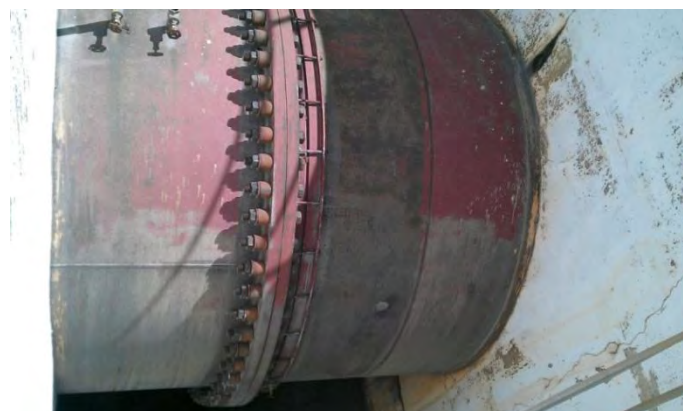
Figure 20: CW duct covered in concrete (PS-01)
