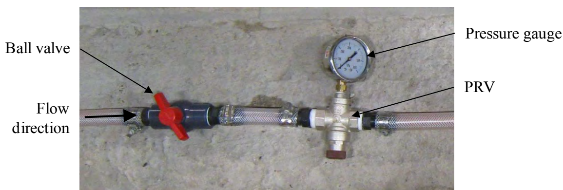
Figure 3.8: Setup of Ball valve and PRV with attached Pressure gauge
