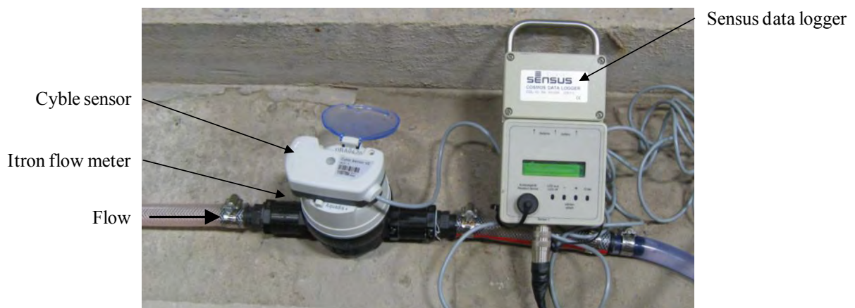
Figure 3.7: Itron flow meter with attached Cyble Sensor and Sensus data logger
