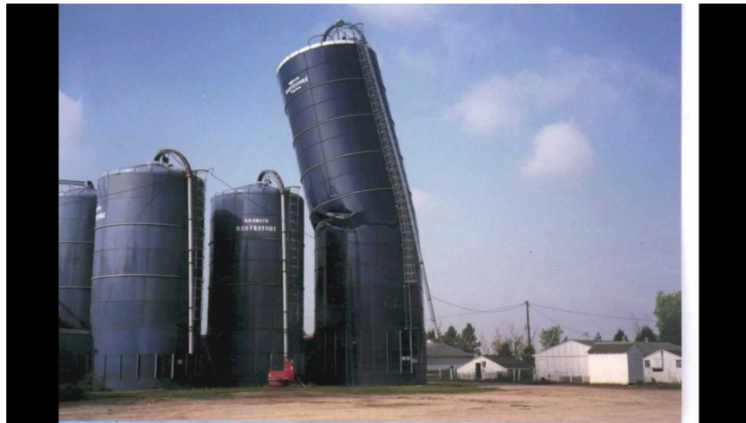
FIGURE 1.3: Silo Collapse. Photo taken from Silo failure video ( https://www.youtube.com )
