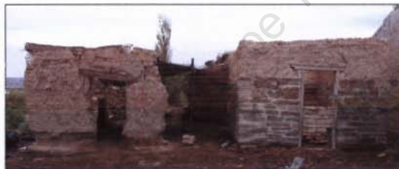
Figure 4.55. Krabfontein. Badly deteriorated brick walls of the extension buildings.
