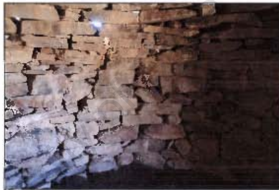
Figure 4.21 De Brak. Cracking, unstable wall caused by running joints.
