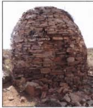
Figure 4.18 De Wilg. The outer layer of the wall has not been tied to the inner layer and is consequently peeling away.
