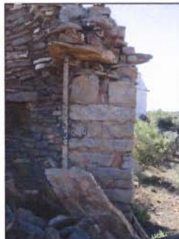
Figure 4.13 Spoorolk. The linking stone can be seen spanning the width of the wall.
