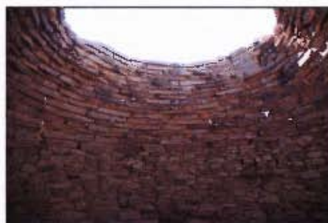
Figure 4.22 De Kolke. The centre of the roof has collapsed.
