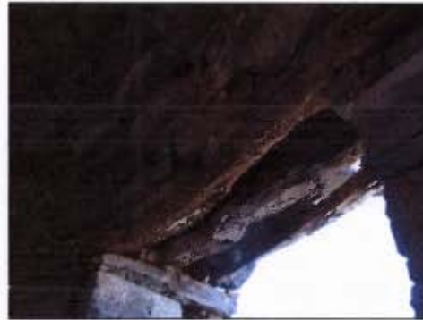
Figure 4.20 Stuurmansfontein III. The wooden lintel is beginning to bend.
