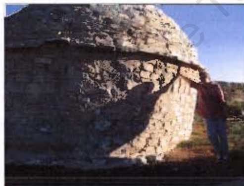
Figure 4.16 Rietpoort. Poor foundations have resulted in this building leaning to one side.
