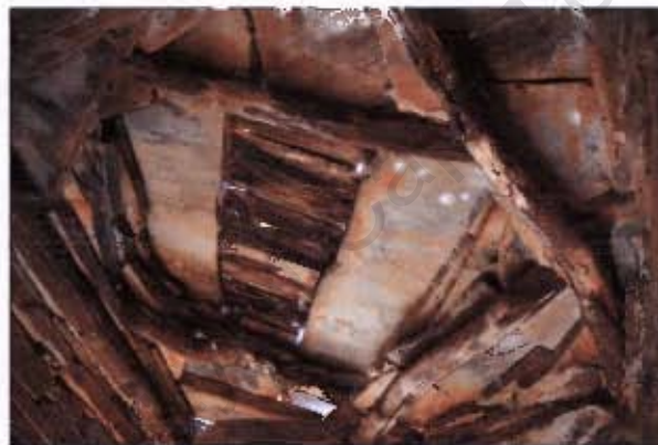
Figure 4.24 De Val. The roof hole is large and timber supports have been used to support the roof stones.
