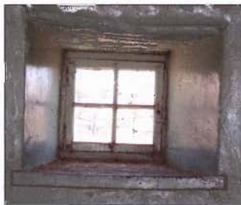
Figure 4.60 Konka. Old glass in the window frame.
