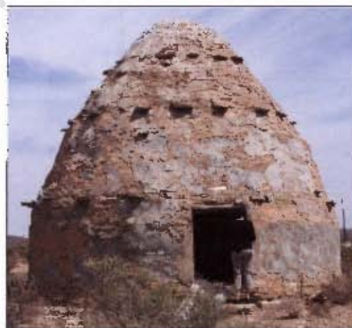
Figure 4.41 Slingersfontein. Remnants of exterior plaster and paint are still present.
