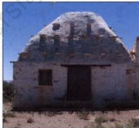
Figure 7.3 Klipkolk. Large square base building which required a particular skill to build.
