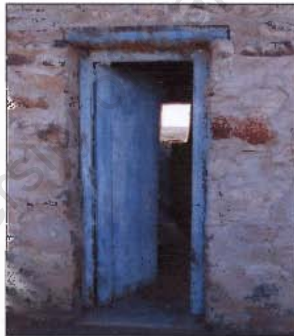
Figure 4.52 Janklaasleegte II. A piece of railway track has been used for a lintel.
