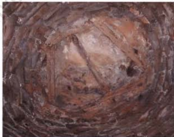
Figure 4.49 Krugerskolk. A miscalculation at Krugerskolk required a timber structure to support the roof stones.
