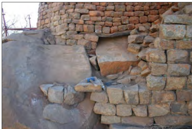
Figure 3.5: Drystone wall construction at Khami also incorporated other materials to stabilise the uneven surface. Here, wood was used to create an even surface across a boulder on the Cross platform.
