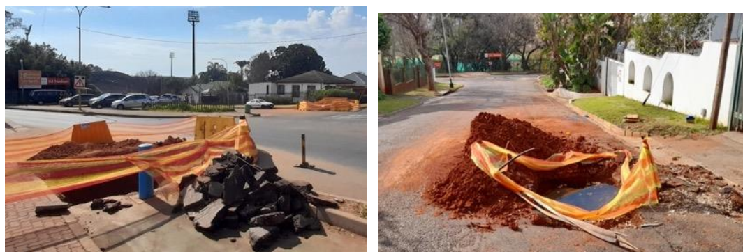
Figure A-38: Road excavations that were fenced adequately (left) and poorly (right)
