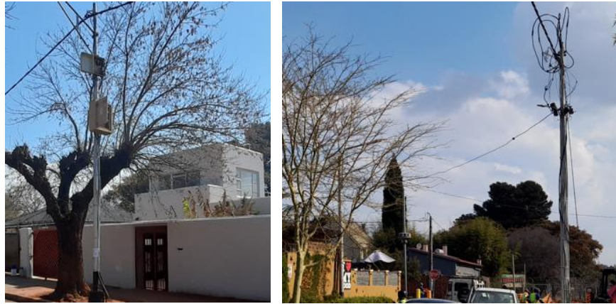
Figure A-36: Vandalised/tampered boxes atop utility power poles with connections leading to private student housing (left) and local businesses (right)
