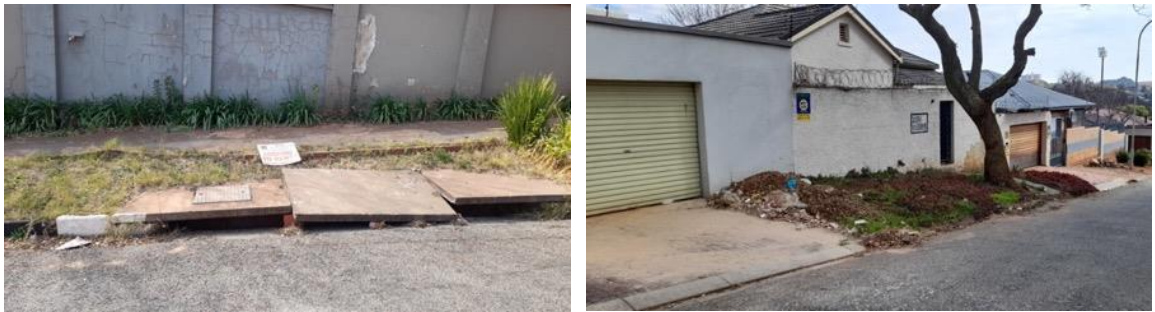
Figure A-34: damaged and/or unkept pedestrian walkways
