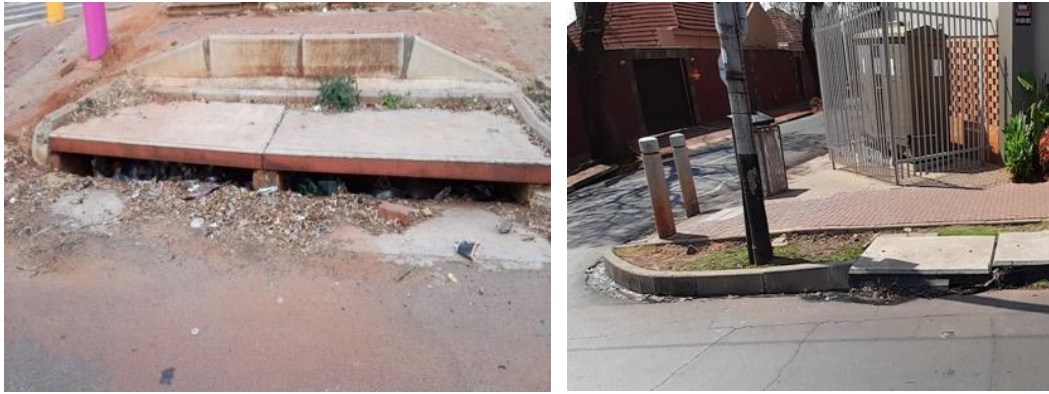
Figure A-33: Drains clogged by litter (with water seeping on the right)
