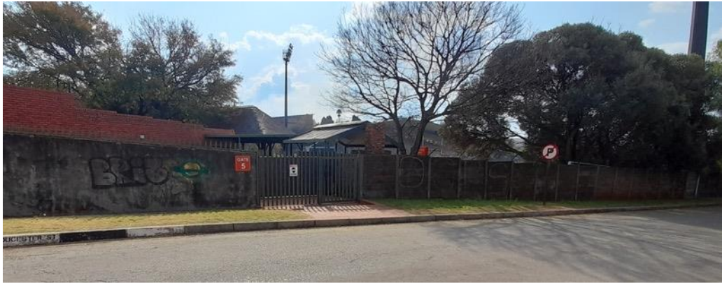
Figure A-30: Graffiti on UJ student facilities' walls
