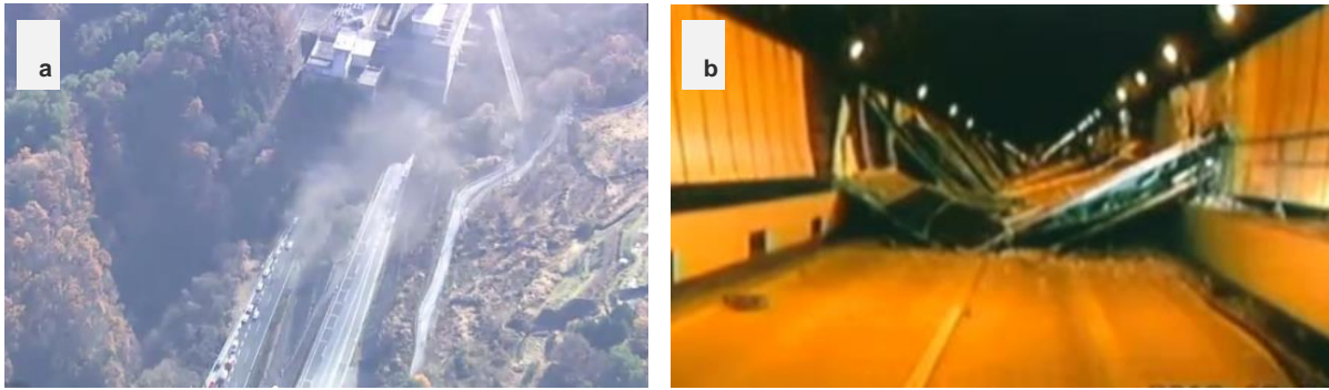
Figure 1-1: Sasago tunnel collapse in Tokyo, 2012 (a) aerial view and (b) inside the tunnel
