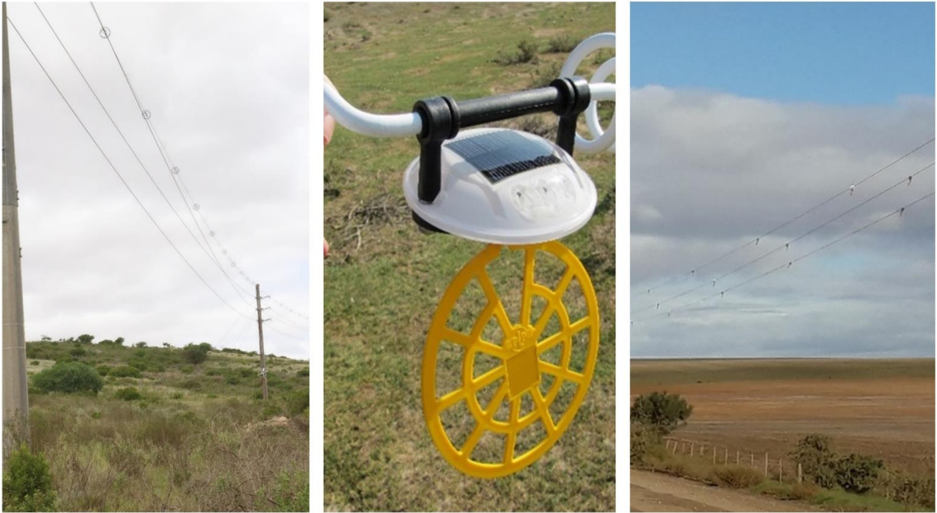
Figure 4: Collision mitigation on powerlines in the Overberg: stationary devices (spirals) (left, photo: Heather D'alton) dynamic device/flapper with an LED (centre, photo: Matt Pretorius) and dynamic devices (flappers) (right, photo: Christie Craig).
