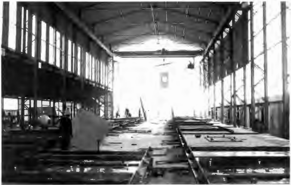
"MUST" SYSTEM - (a) Inside the Philippi factory, showing casting tables & the overhead gantry.
