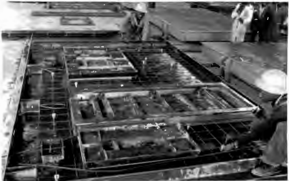
"MUST" SYSTEM - (b) Steel door and window-frames and reinforcing steel in position ready for casting an exterior wall panel.
