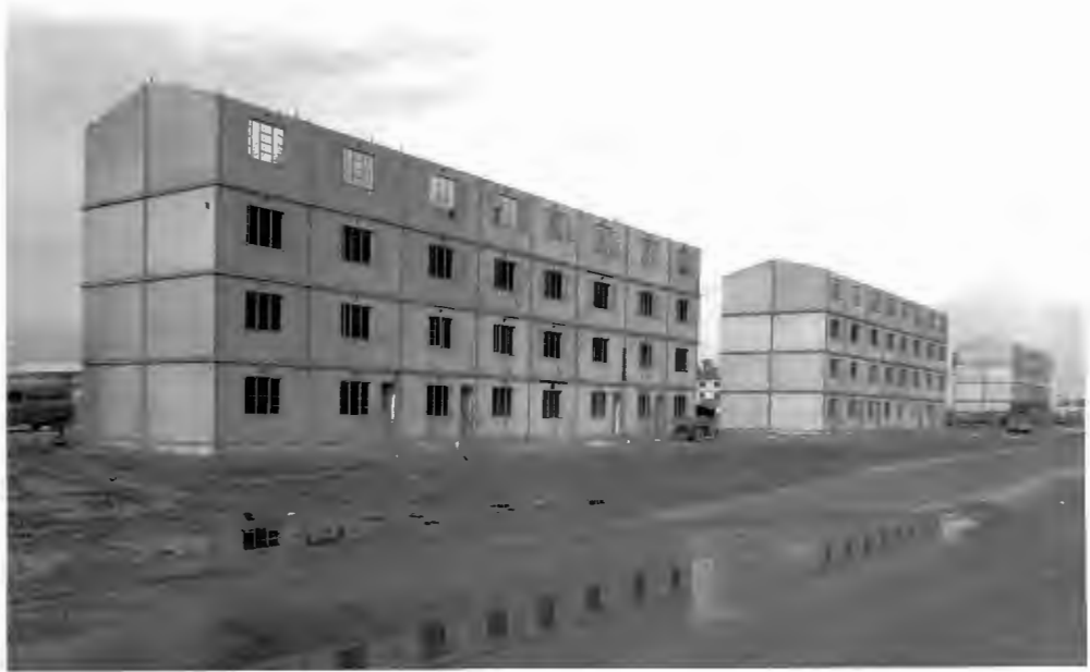
"MUST" SYSTEM - (j) Blocks of flats, showing precast panels erected to four storeys.
