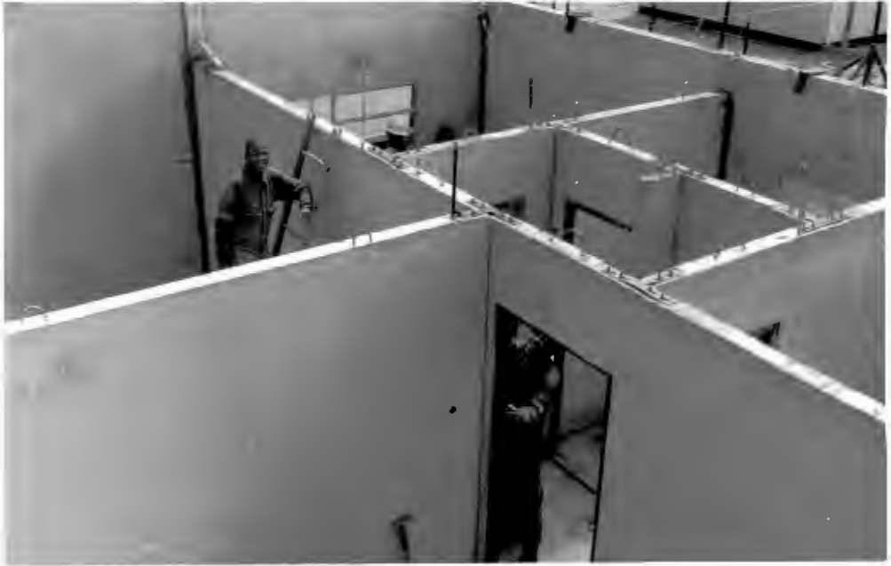
"MUST" SYSTEM - (i) The assembly of interior wall panels showing lifting hooks, tee joints and electrical conduit cast into the walls.
