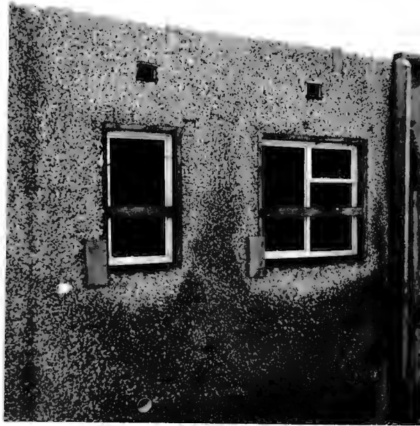
An exterior wall showing window frames cast in position; the open texture of the concrete can be clearly seen.
