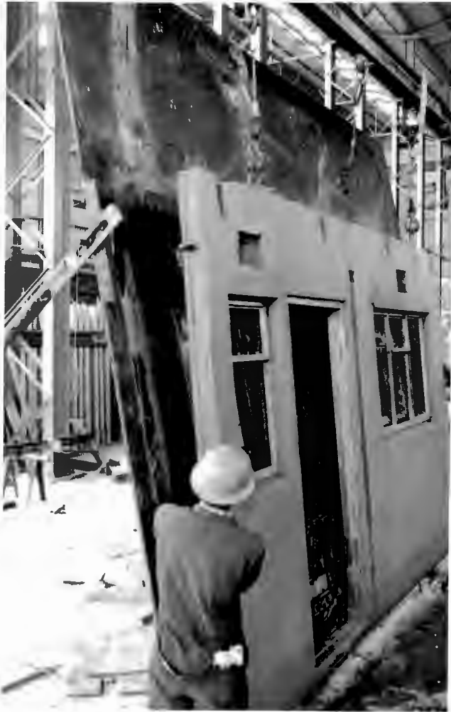
"MUST" SYSTEM - (e) Casting table tilted to near vertical and panel being lifted clear.
