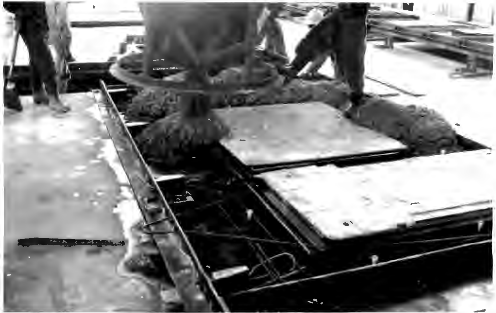
"MUST" SYSTEM - (c) Concrete being placed in the wall panel on the horizontal table. Door and window frames are temporarily masked.
