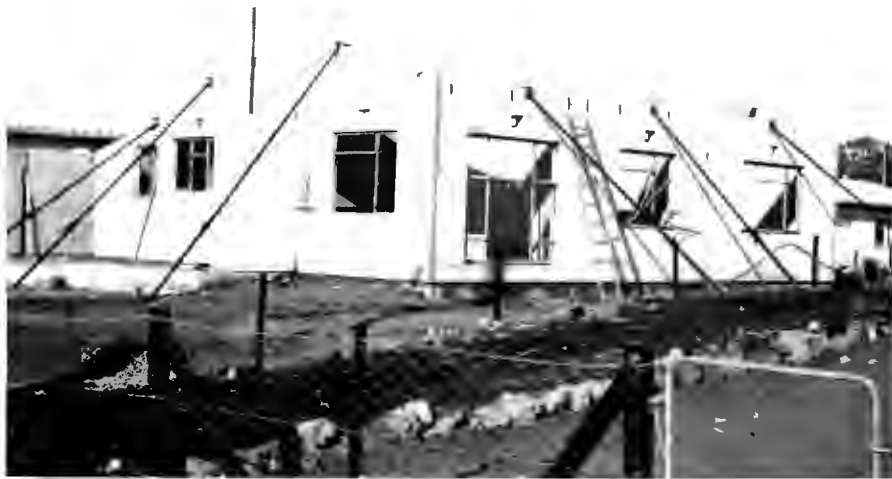
"MUST" SYSTEM - (h) Erection of walls completed; temporary props in position while tee joints are made & roof trusses positioned in the slots shown.
