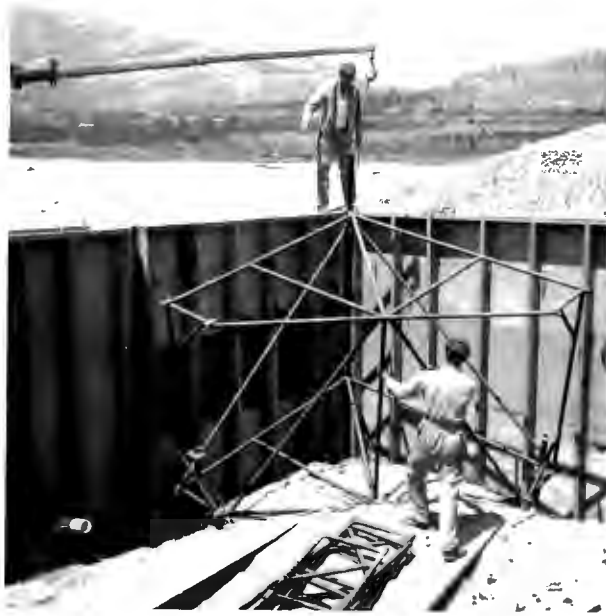
Removing the internal jig bracing prior to stripping formwork; the light construction of the formwork can be seen.
