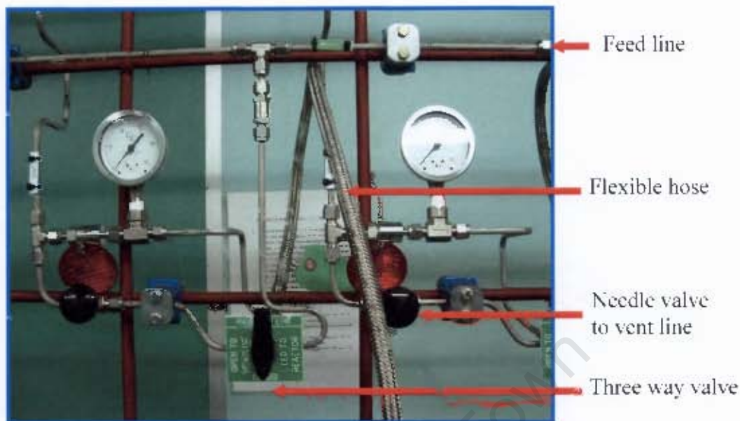
Figure 4.4: Picture of flexible hose, three way valve and supply/vent line.
